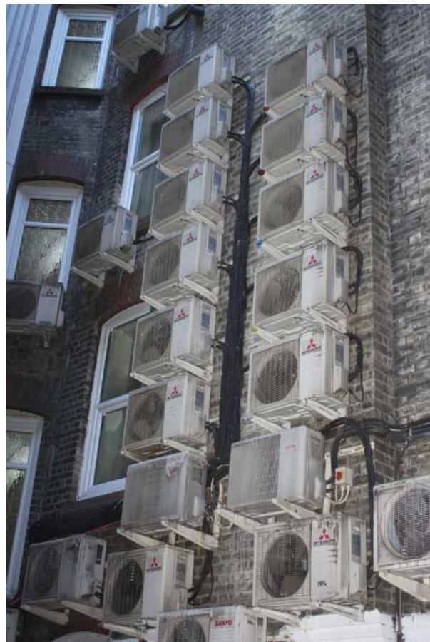
Figure 3: Existing hotel external a/c units
