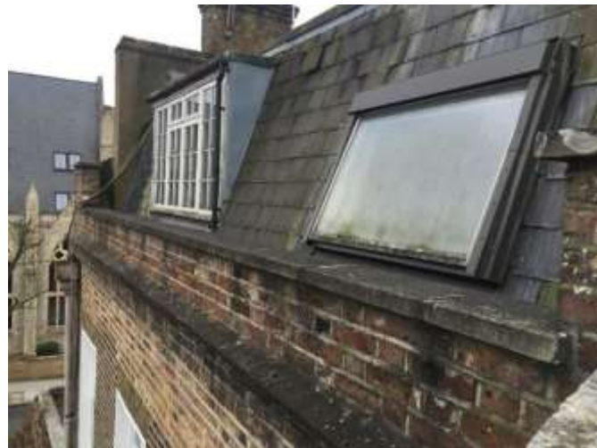
Fig 79: Lower quality coping and parapet extensions at ends
