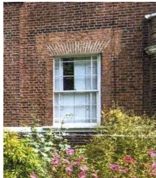
Fig 70: Patchiness from removed stucco
