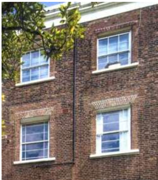
Fig 69: Inconsistent windows and brick arches
