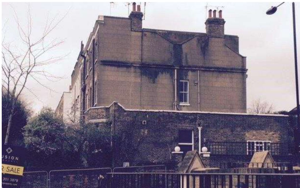
Fig 41: South elevation showing staining of concrete render after rain
