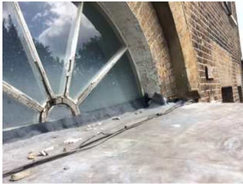
Fig 68: Glazing bars on the fanlight showing deterioration
