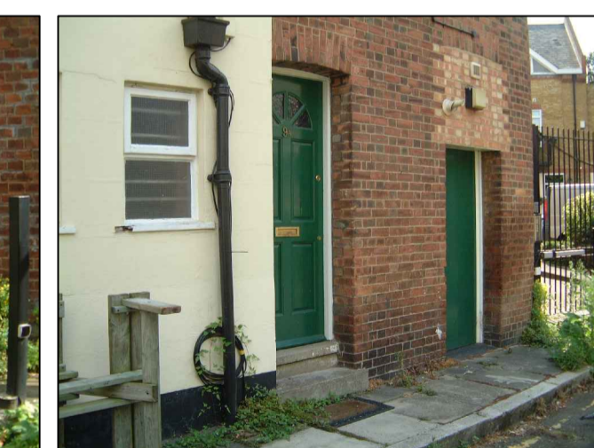
PHOTO INDICATES HEAD OF EXISTING DOORWAY BRICKED UP WITH NON MATCHING BRICKS INCLUDING EXTRACT VENT TERMINAL, BOILER FLUE AND BULKHEAD LIGHT FITTING
