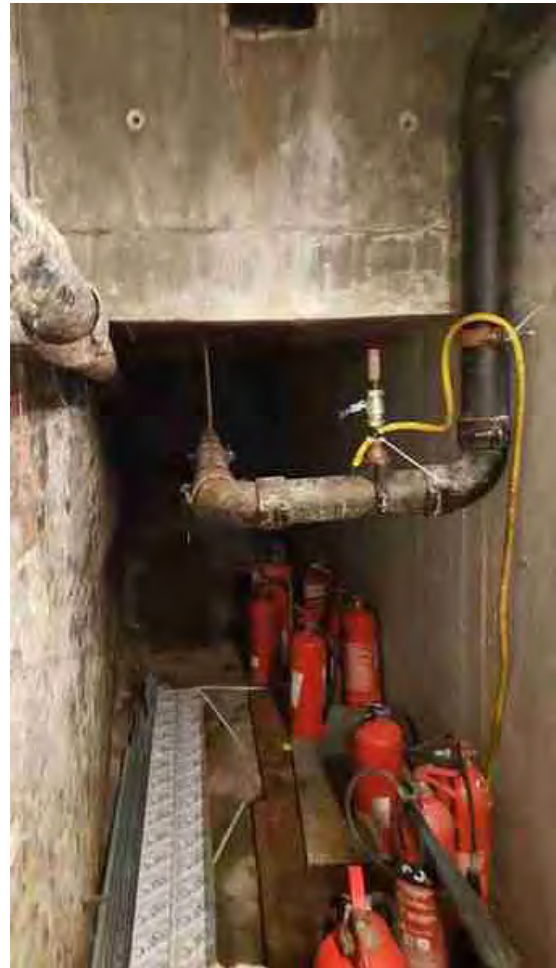
Photo 2: View of rear of the subterranean space between Holiday Inn and 51 Calthorpe Street.
