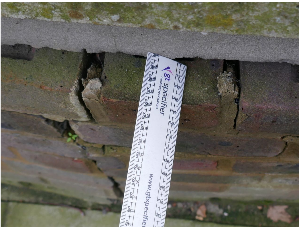
4) Lateral displacement just under 30mm
