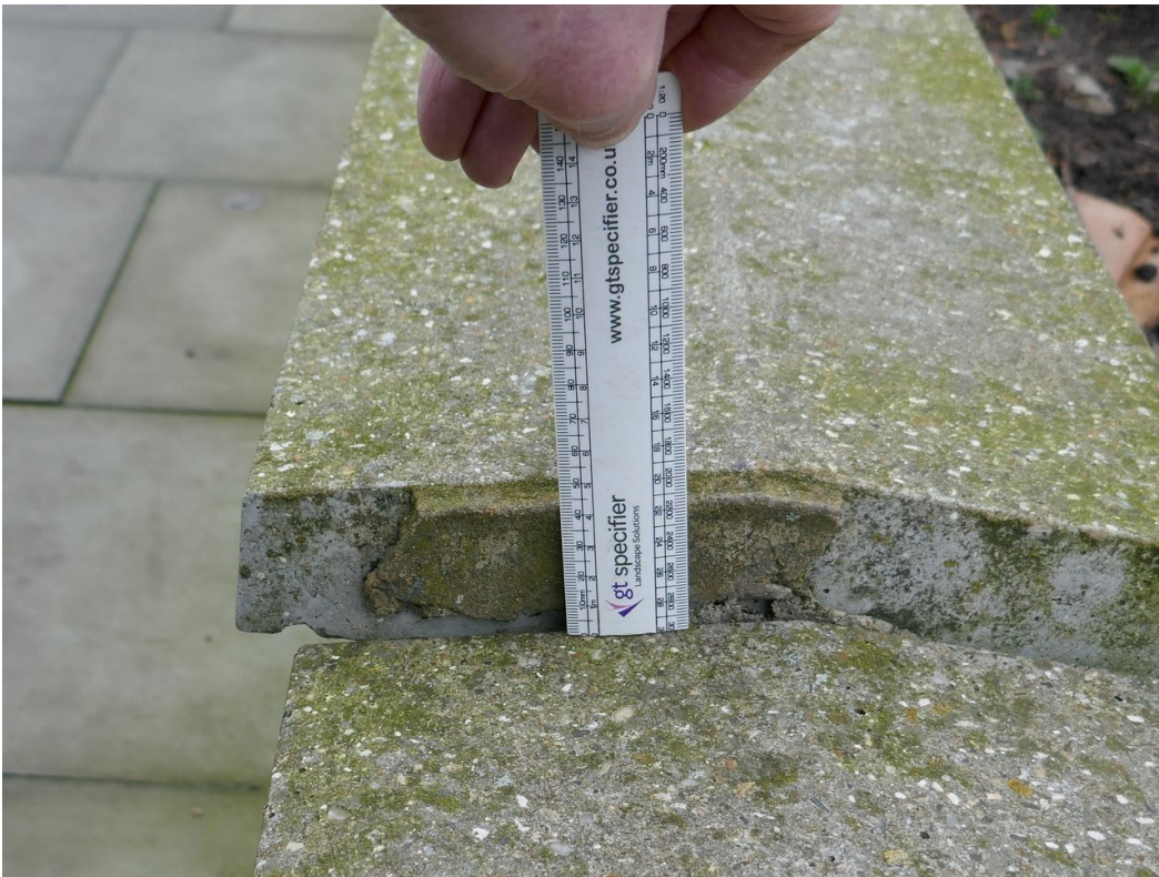
3) Vertical displacement about 50mm
