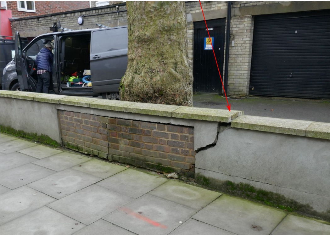
2) Wall in February 2017, damage noticeably more severe, as more of the end of the lifted section is visible.
