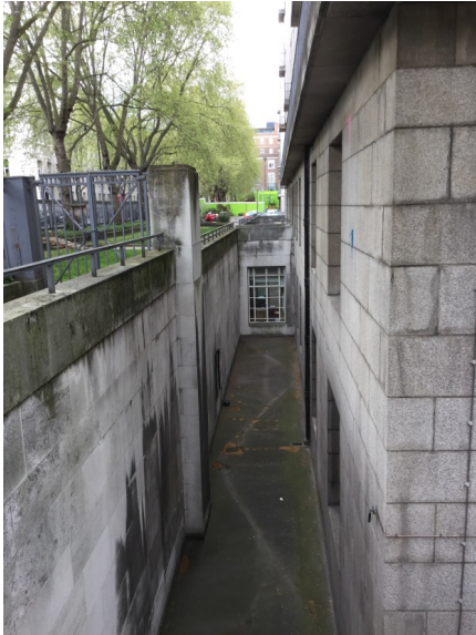
Photograph of the existing Light-well to Senate House South Building facing Malet Street.
