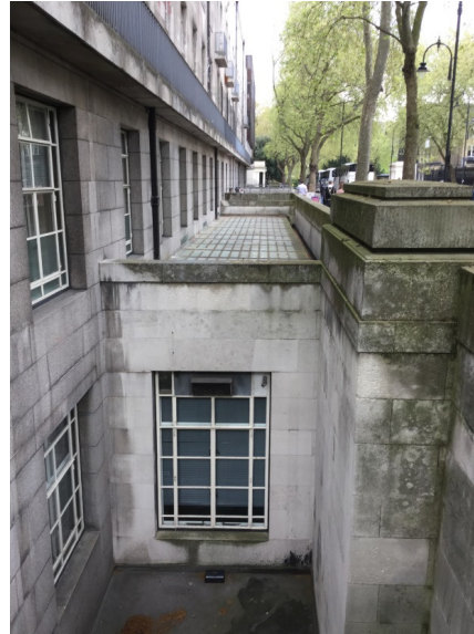
Photograph of the Charles Holden In-filled Light-well to Senate House South Building along Montagu Place.
