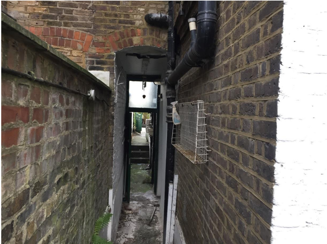
Photo 5: walkway door and window to be replaced
