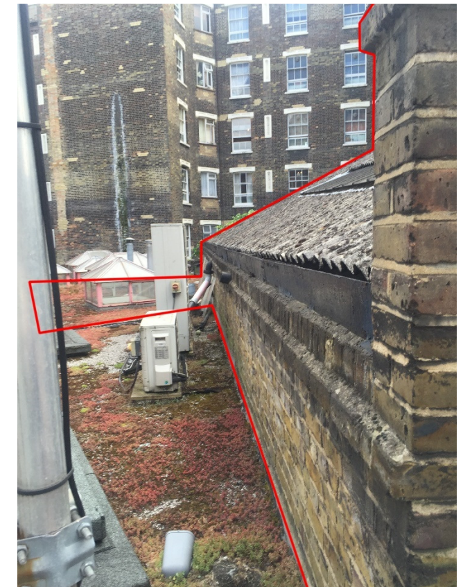
Site Photo 4 Exterior of the Land to the rear of 159-163 Kings Cross Road (East Boundary) Photo facing South
