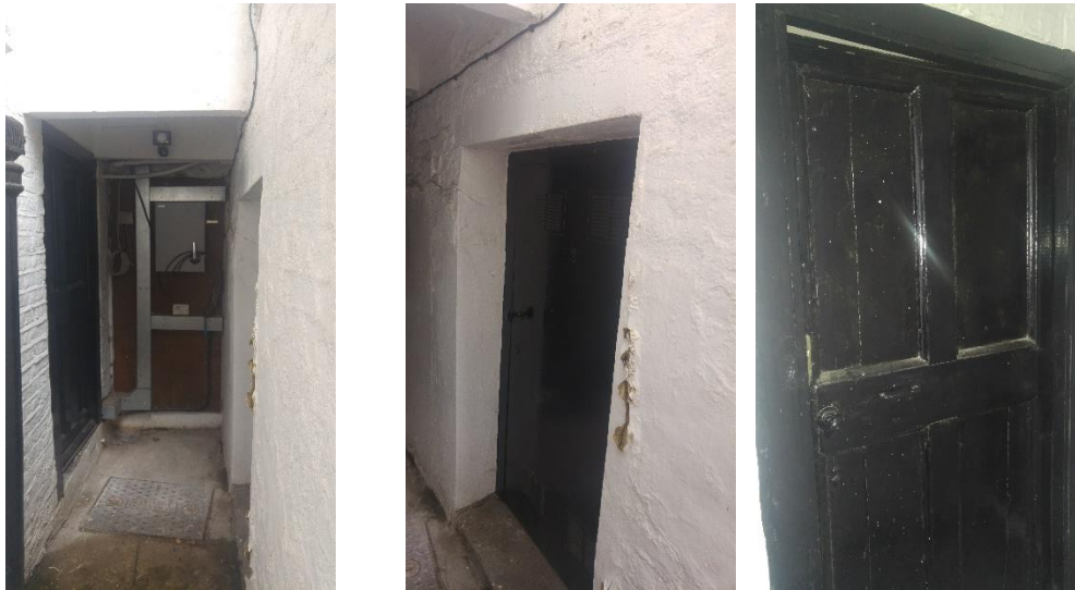
View towards basement front door Vault room door to be narrowed Basement front door
