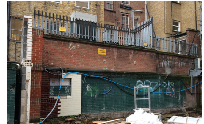
Ad hoc development with a series of utilitarian flat roofed back extensions vary in height and materials.
