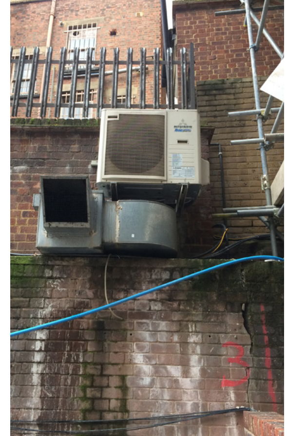
Mechanical plant fixed to party wall with 43 Leather Lane.
