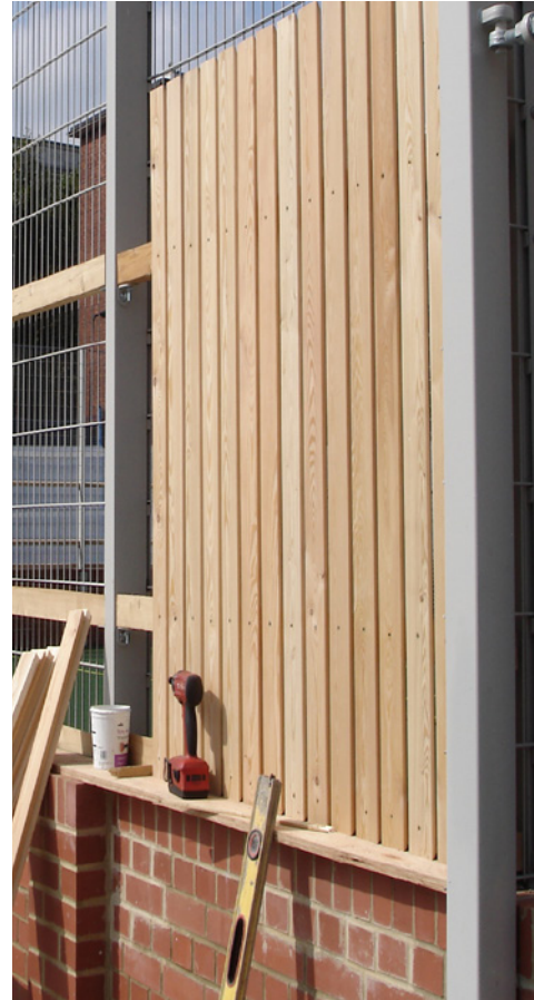
Larch vertical fencing on garden wall bond, brick on edge capping. MUGA detail.
