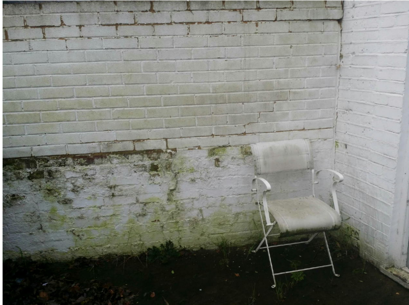
Photo two: shows left hand boundary wall with cracking. Lower section is 225 mm thick brickwork; the upper more modern section is 100 mm thick.
