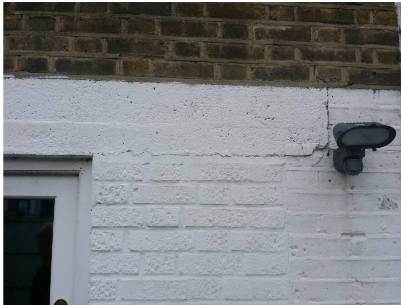
Photo three: shows cracking around the right-hand bearing of the main lintel.
