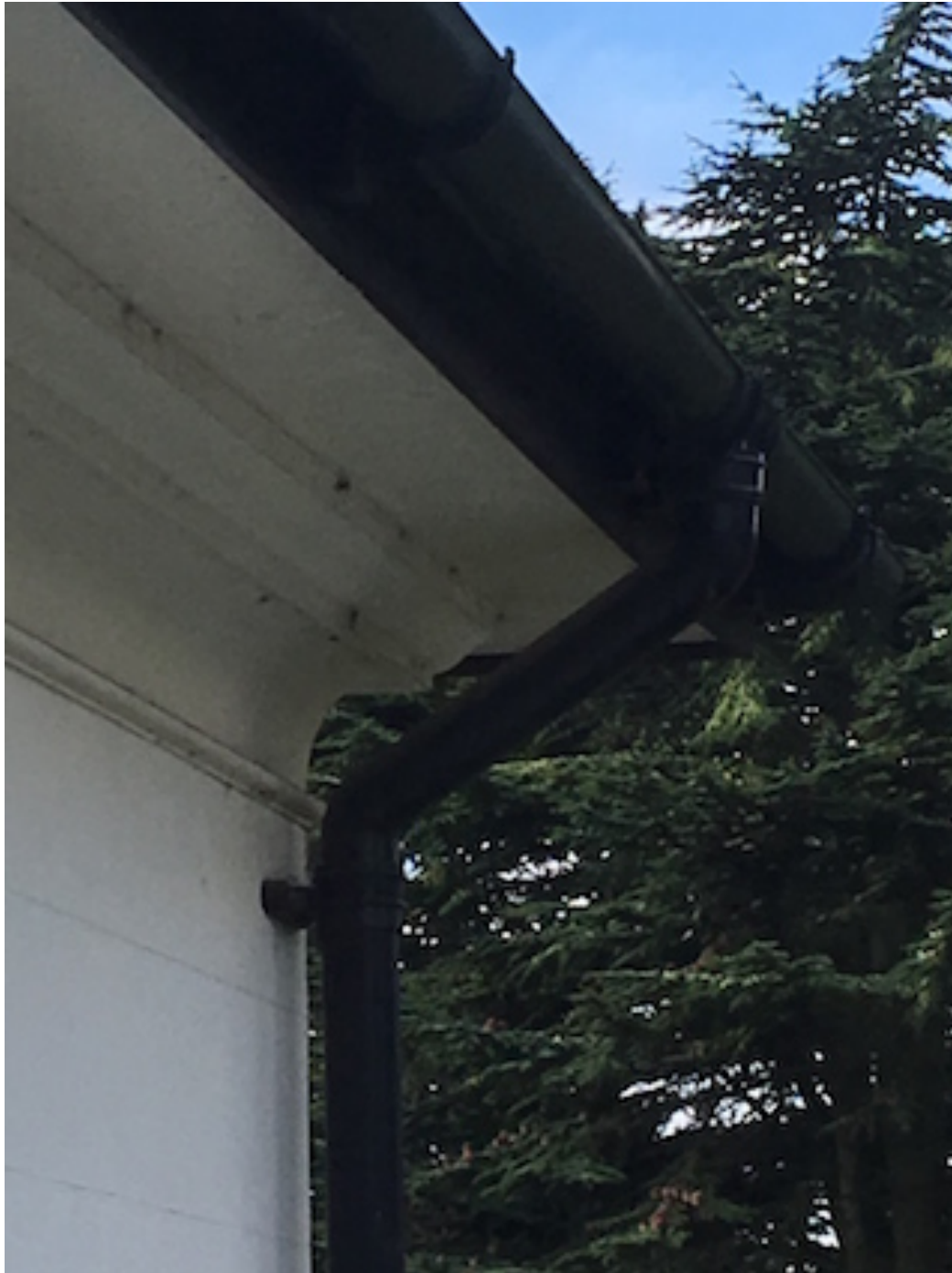
Photo.2 Example of the as installed rainwater gutter and pipework due for replacement. (Oct 2016)
