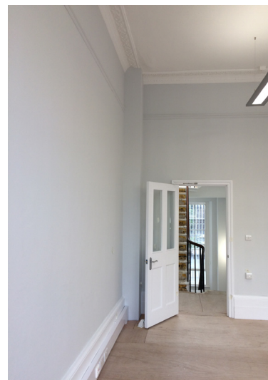
Typical riser location as installed
