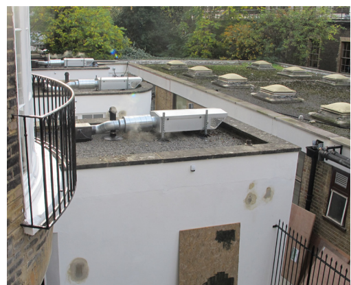
External Mechanical services / railings as installed
