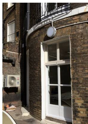
External lighting as installed
