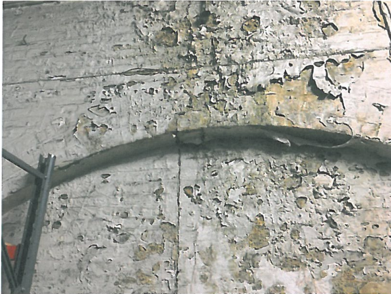
Sample 03 – Flaking paint to wall – No asbestos detected.
