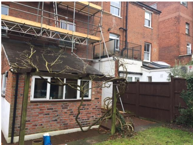
Photo 5: View of existing single storey rear extensions at Nos. 8 and 6 Nassington Road
