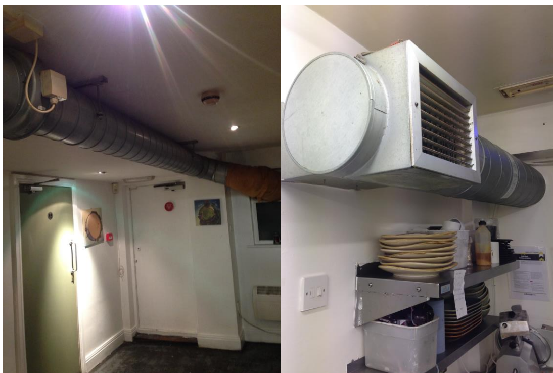
Image 5.1: Installed Extraction System
