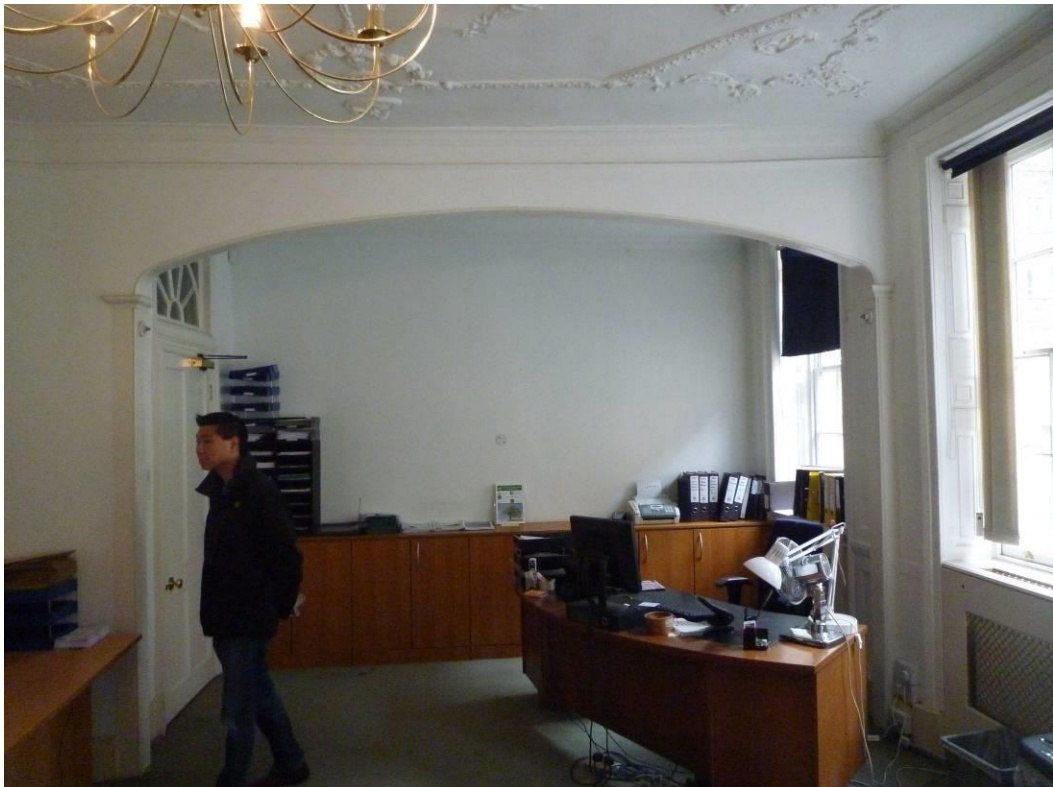
Fig.38 Ceiling in first floor front room from the north, showing the modern archway (AHP)
