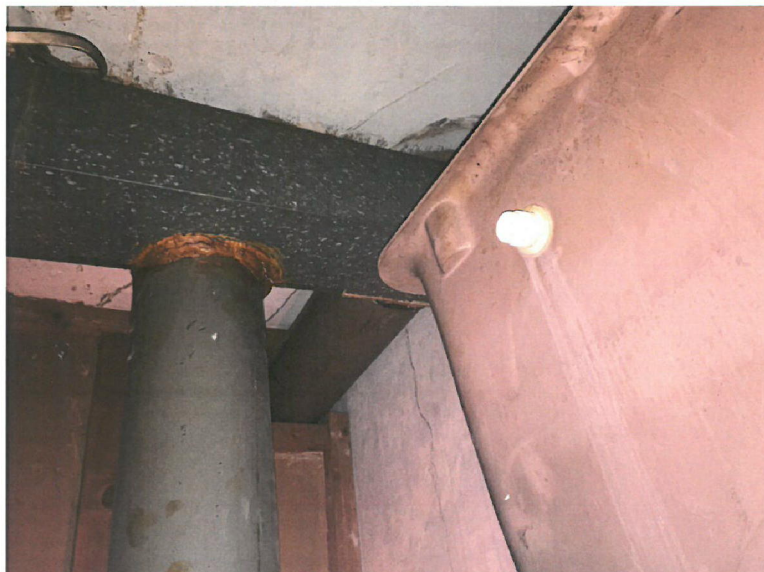
Photo D – Air extraction / ventilation ducting within suspended ceiling located within Bathroom.
