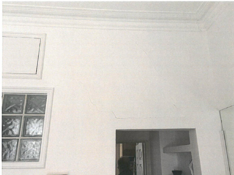
Photo C – Cracking to internal load bearing wall appears to have spread, crack widths have remained static.
