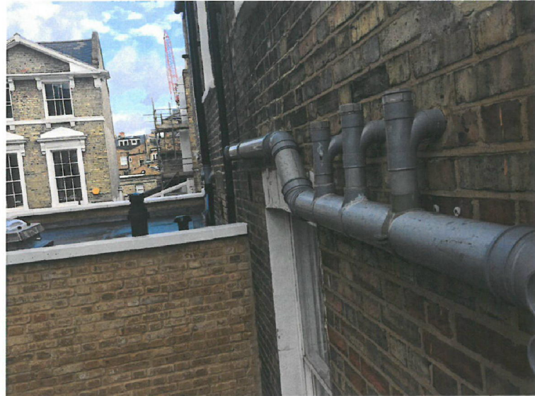
Photo E – Existing assumed foul water pipework from 2 nd floor flat to be relocated.
