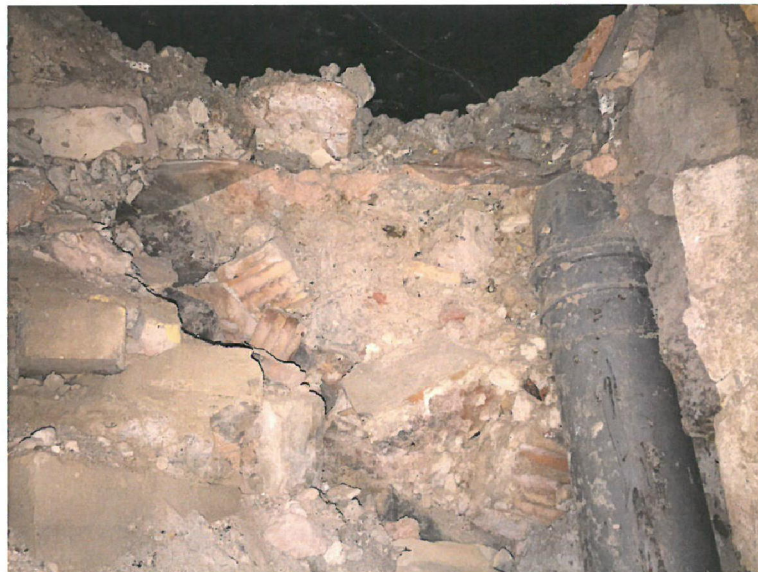
Photo B – Rainwater pipe and underside of slab to butchers preparation area.
