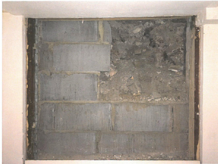
Photo A – Blockwork removed from window / coal chute revealing construction rubble material.
