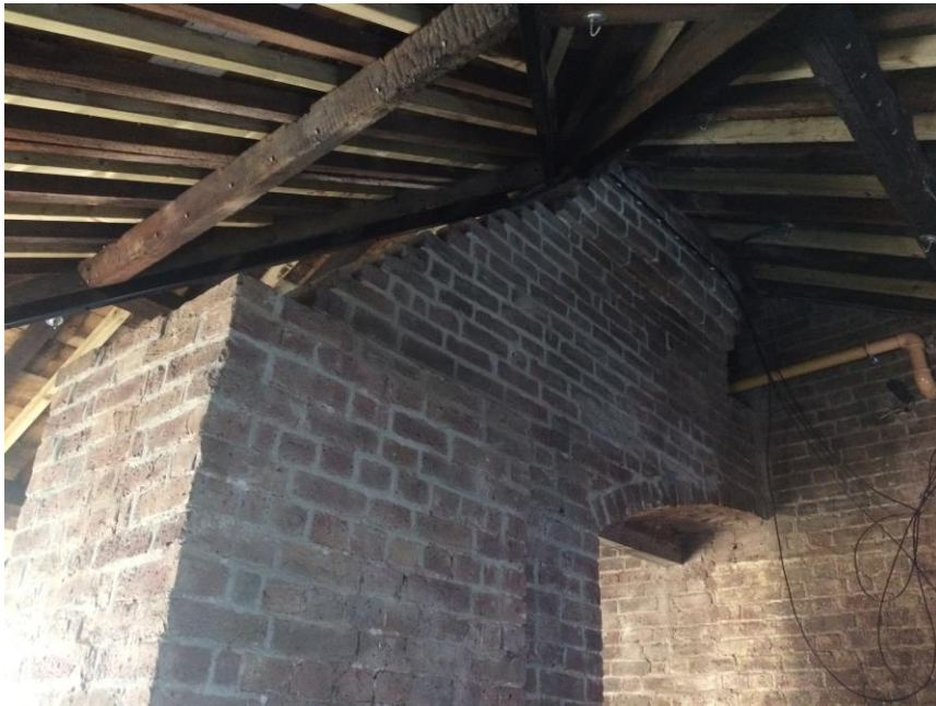
Figure 11: Chalk Farm Building, first floor: view from south room (unit 38) showing repaired roof structure. A plaster finish ceiling sloping soffit will be reintroduced to the joist underside.
