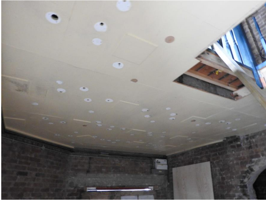
Figure 13: Chalk Farm Building, ground floor: existing modern ceiling – modern, poor quality plasterboard, with marks and holes from the previous tenant.
