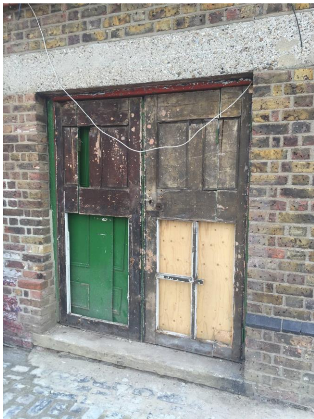
Figure 15: Chalk Farm Building, west elevation, external folding door to right hand side: the doors are of some age, but reused from elsewhere, cut a quarter in down their length and hinged, turned upside down and then lined each side with odd facings.
