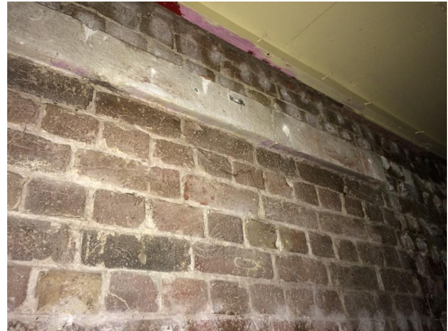
Figure 12: Chalk Farm Building, ground floor: view of north wall high level (unit 39) showing the projecting horizontal stone course the purpose of which was to provide for sufficient fixing for the rolling/sliding external site entrance gate (refer to fig.5).
