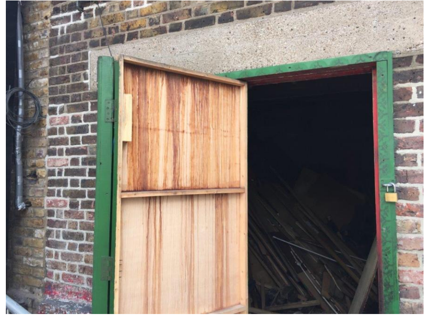
Figure 14: Chalk Farm Building, west elevation, external folding door to left hand side: the doors are modern poor quality plywood.
