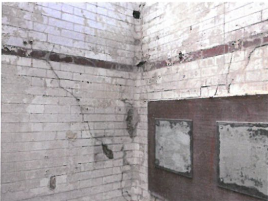
Severe structural crack, wall paint on tiles
