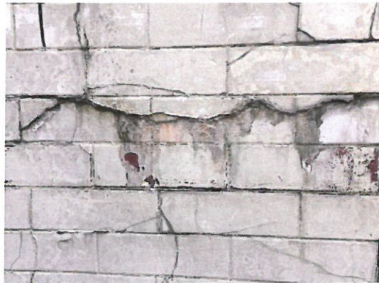
Exterior wall, severe movement and moisture ingress
