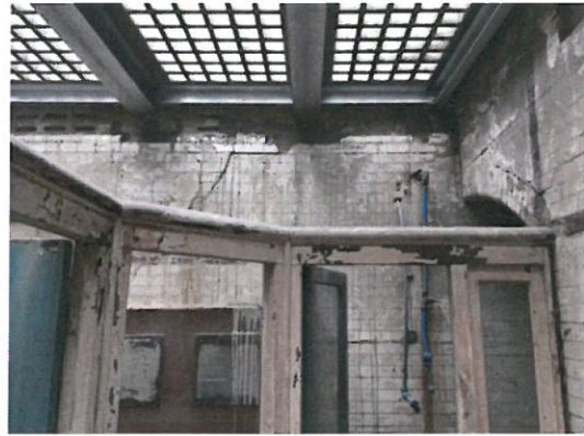
Generally in better condition than Gents Toilet, Repairs required at high level
