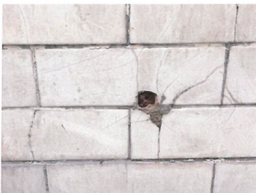
Impact damage, previous wall fixing damage
