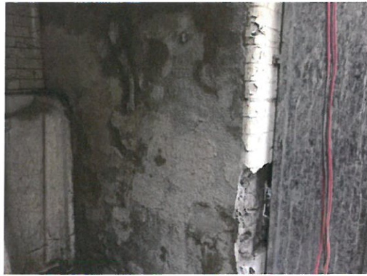
Large rendered section, missing tiles
