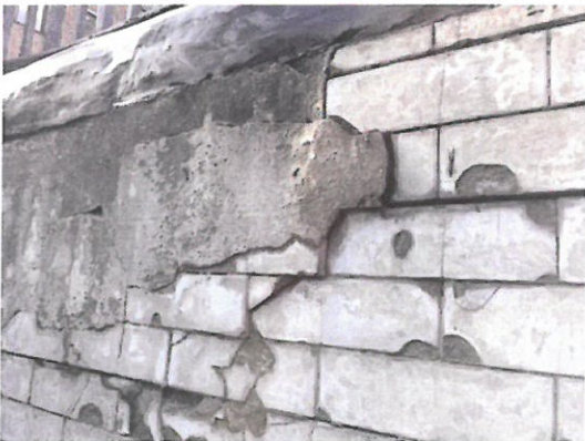
Exterior wall, previous unsympathetic repairs, indicating historic structural failure
