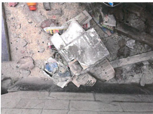
Detached sections from vulnerable areas at high level
