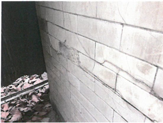
Structural failure, horizontal crack
