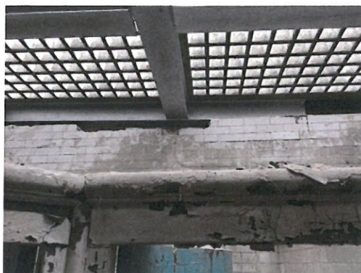
Missing and damaged tiles at high level following reinstatement of new roof light
