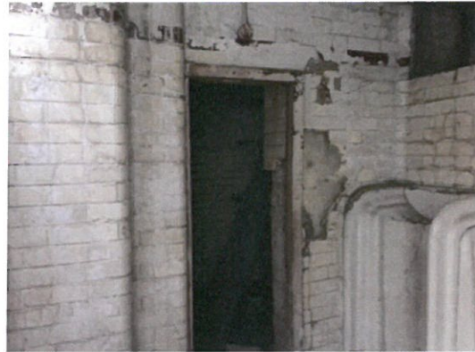
Paint in tiles surface, numerous missing sections
