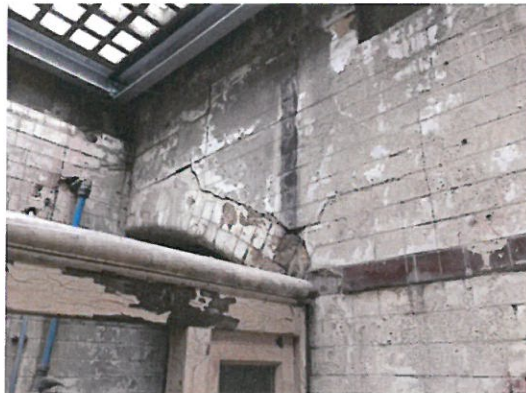
Arched lintel has failed, repaired by pinning or removing and reinstating
