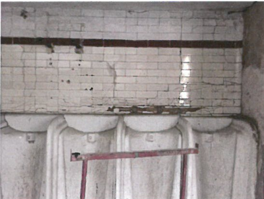
Delaminated tiles above urinals
