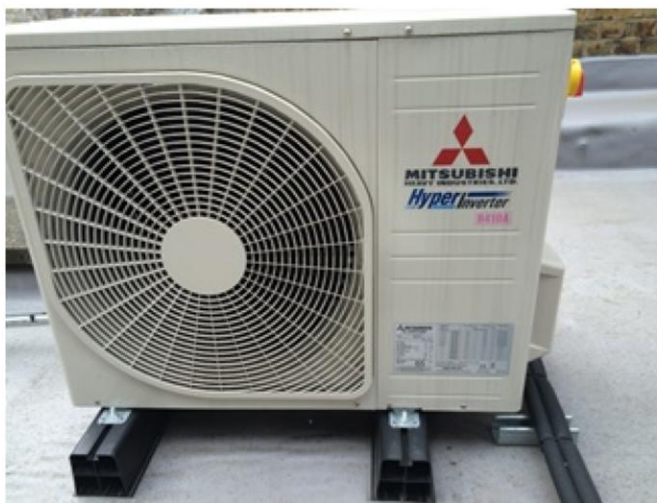
View of Mitsubishi external condenser air conditioning unit.
