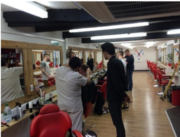
View of inside of London School of Barbering, showing internal air conditioning unit in ceiling.
