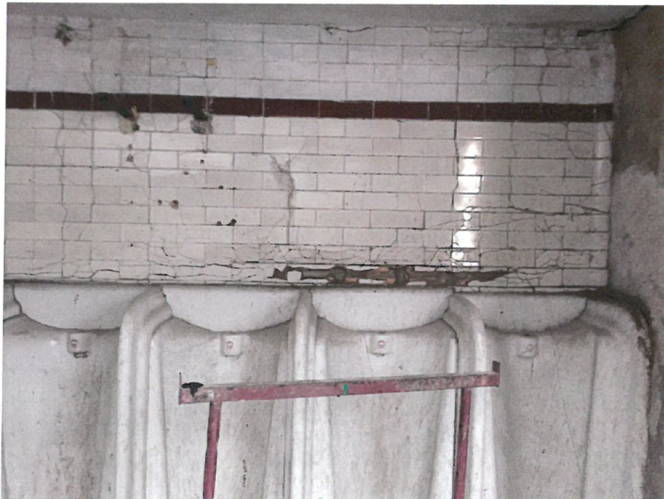
Cream tiles for the majority of the wall areas <2.1M height, then a single brown tile, then white to ceiling height, up to 3.1m.
