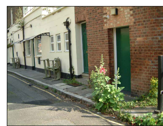
EXISTING WHITE RENDERED WALLS WITH COPING DETAIL TO BE RETAINED NEW OPENING TO BE FORMED IN EXISTING WALLS
