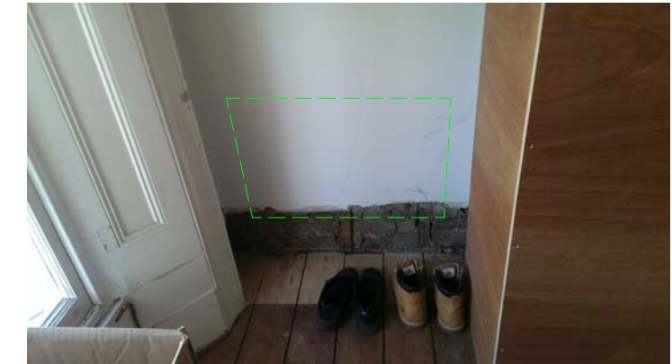
Proposed new radiator location to increase BTU output. Existing plain wall. New notches in joist may be required for new rad positions.
