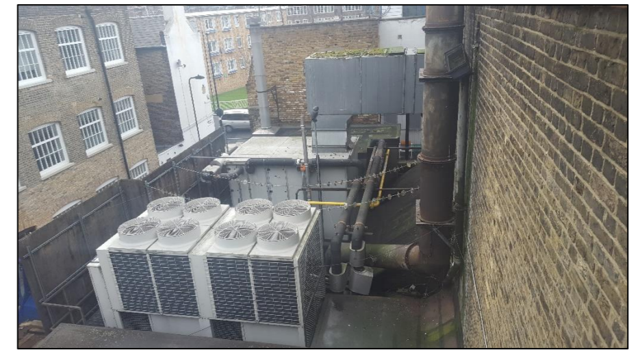
Photo 10: Plant machinery on the roof of B1, towards the north.
