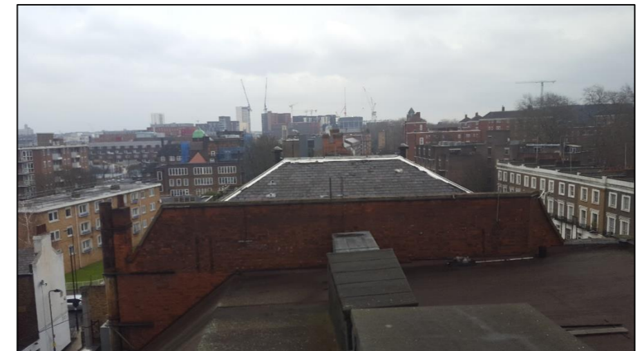
Photo 8: Looking east at the slate tiled pitched roof from the roof of B1.
