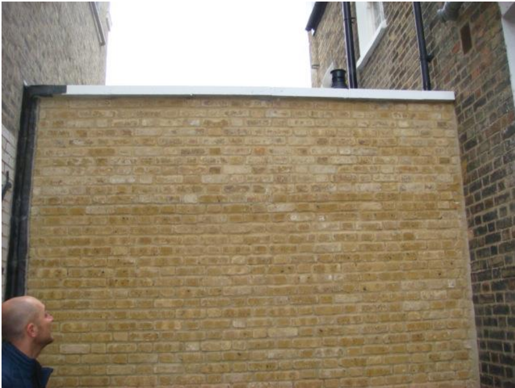
REAR 65 REGENTS PARK ROAD LOOKING EAST (NB - showing wall of new extension to 67 Regents Park Road)
