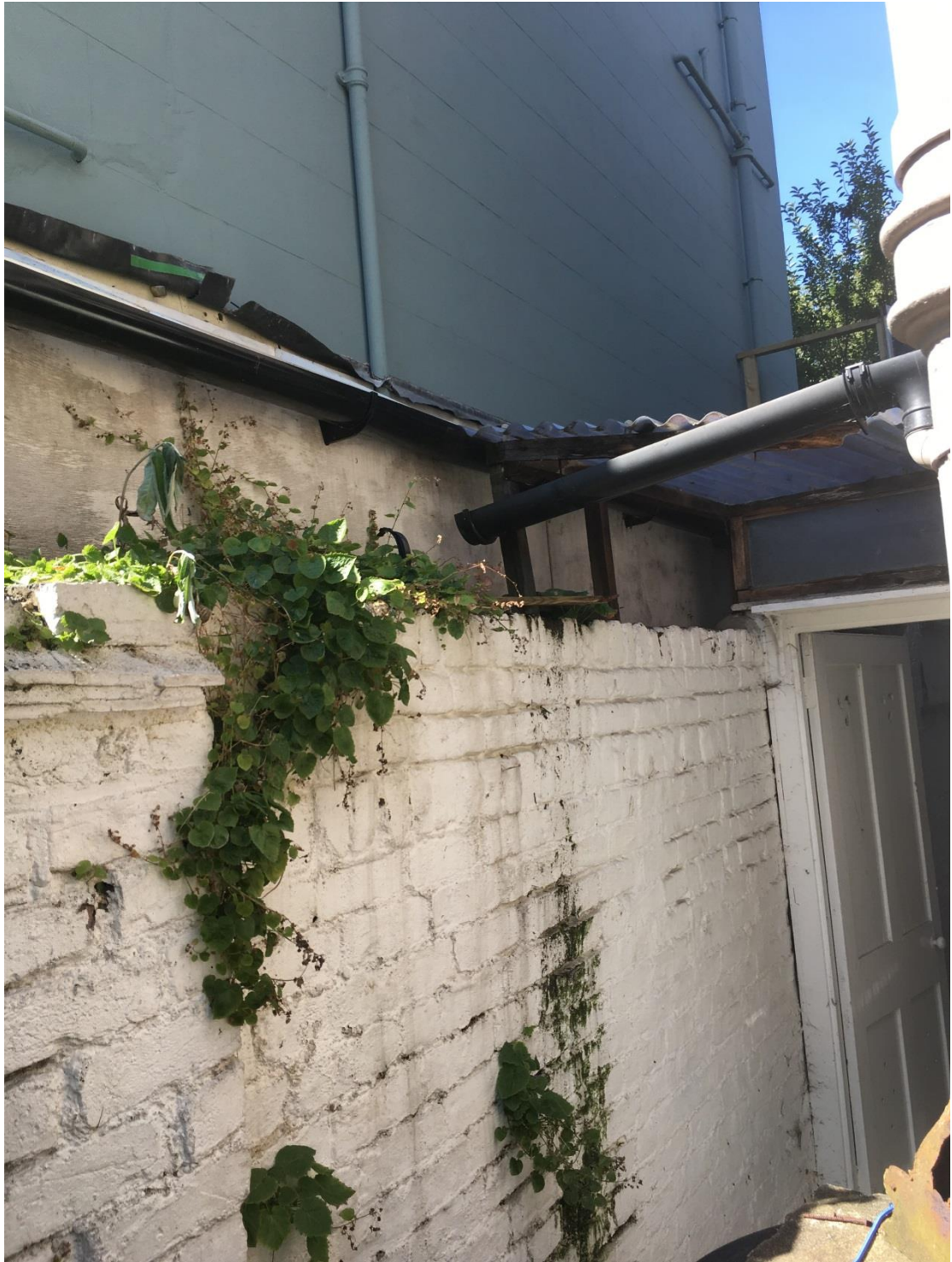
Picture 3 – Existing Lean-to Structure to the side of the existing dwelling house
