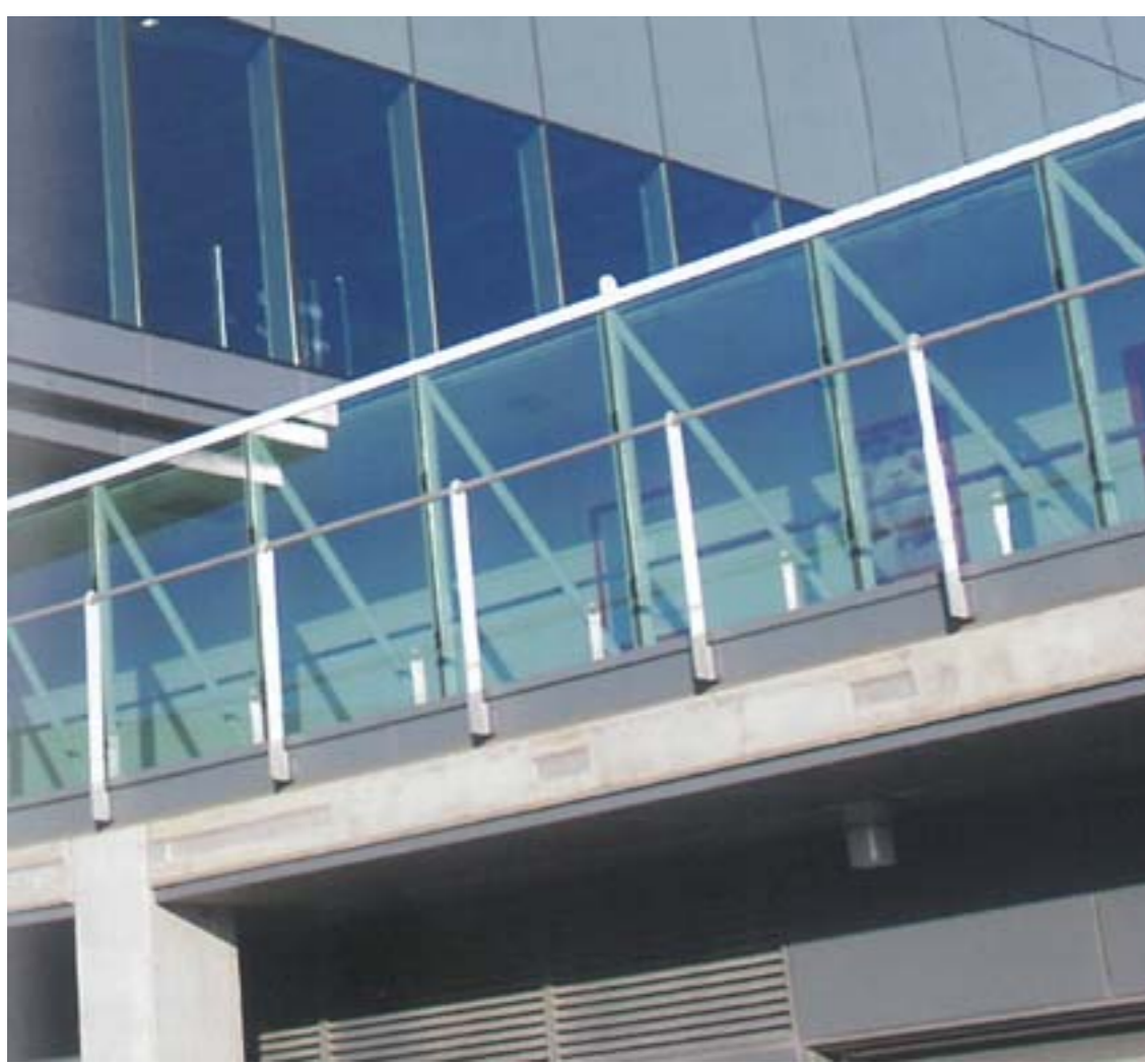
PHOTO: Heathrow PT Slab Edge Detail with Concrete Patching Repair Cement detail.
