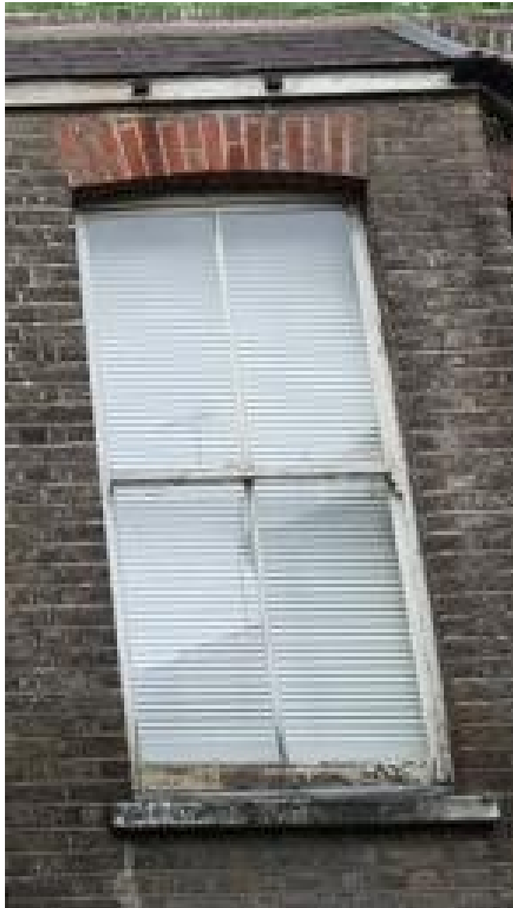
IMAGE 4: Typical dilapidated window
