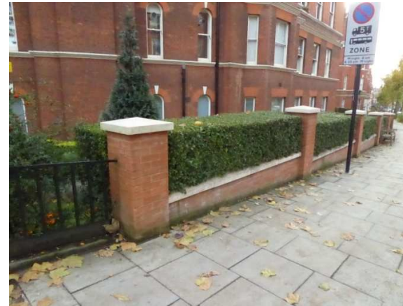
6) View of new section of boundary wall outside Avenue Mansions, at junction with replacement railings fronting Finchley Road.
