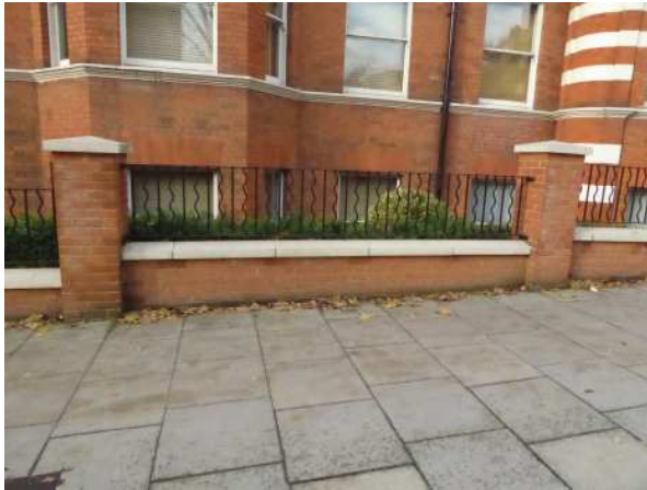
5) View of new section of boundary wall outside Marlborough Mansions. Brick matches main block.
