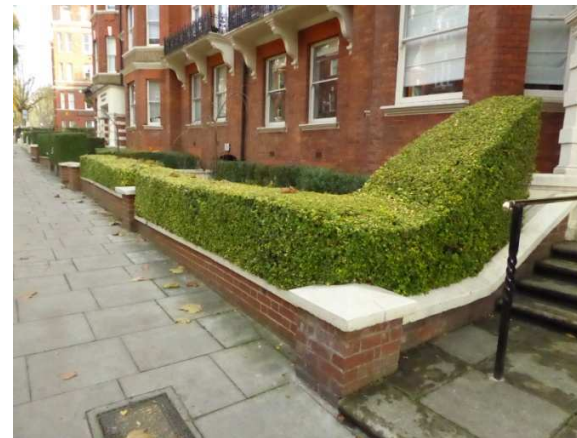
8) Older section of wall, possibly original, which has been reduced in height and capped, following removal of original railings.
