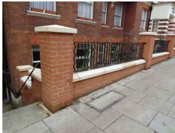
7) New section of wall to one side of the service entrances into Marlborough Mansions.
