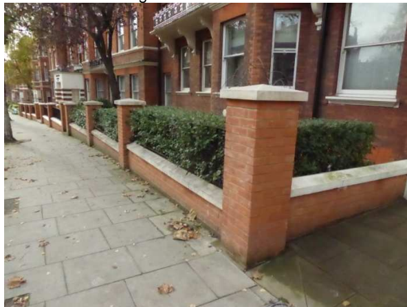
11) View down Cannon Hill showing privet screening to basement flats, behind new railings.
