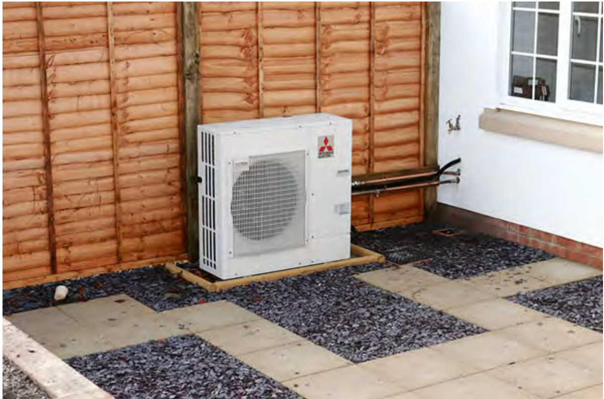
Figure 16 – Typical Air Source Heat Pump External Condenser
