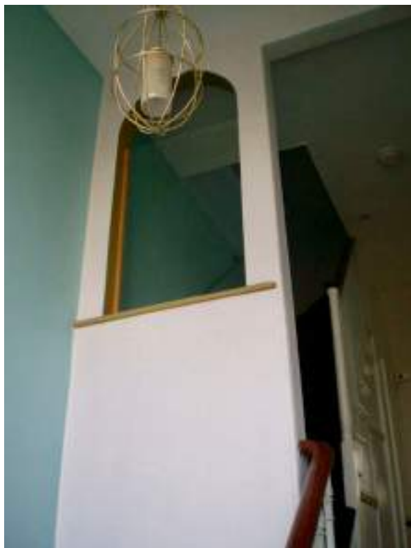
Partition between principal staircase and secondary stairs. Original Feature - High Significance. Arched opening a harmful modern alteration.
