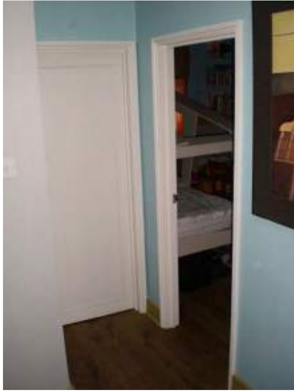
Third floor landing. Overall, Low Significance. Non-original doors and partitions - Harmful modern alterations.
