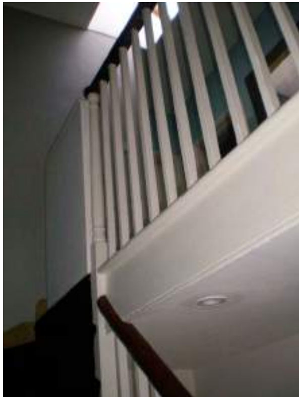
Third floor landing. Original balustrade with turned newel post and stick bannisters - High Significance.
