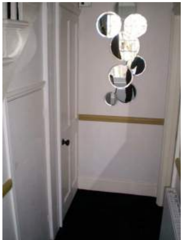
Second floor landing. Airing cupboard and altered partition wall and door position of front room. Harmful Modern alteration.
