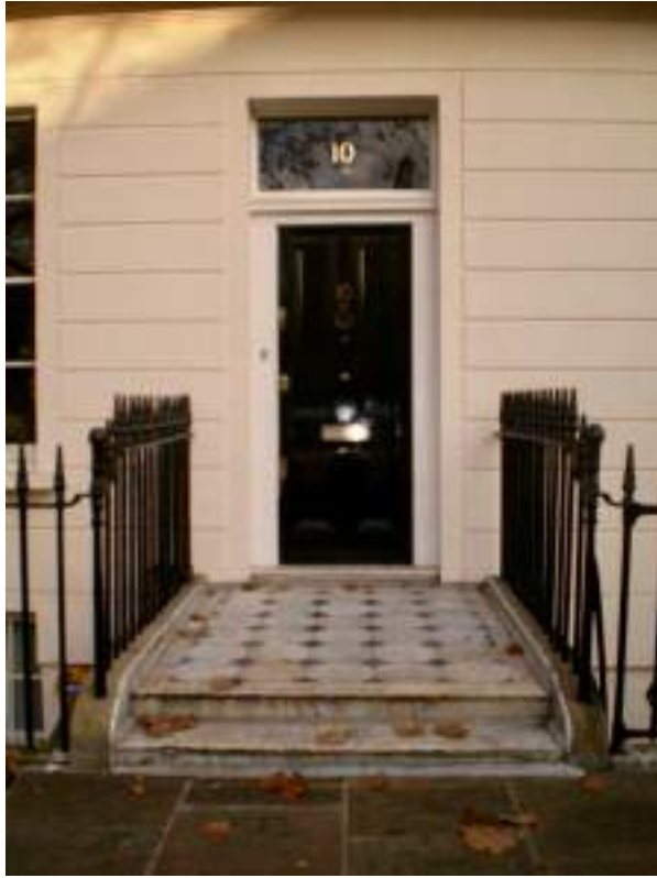
No. 10 Four-panelled door with ogee bolection mouldings - High Significance. Steps and landing clad in marble & marble tiles - No Significance. Harmful modern alteration.
