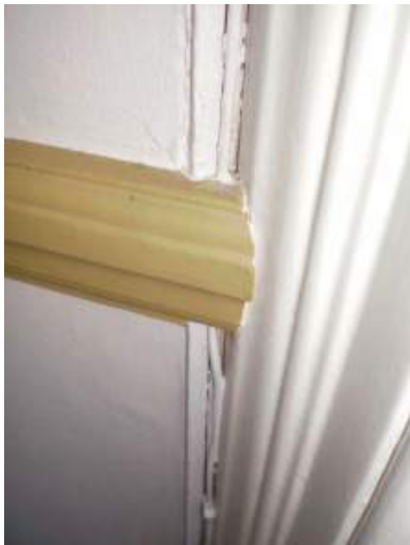
Detail of original architrave of French doors on first floor half-landing - High Significance. Modern dado rail running into it - No Significance.
