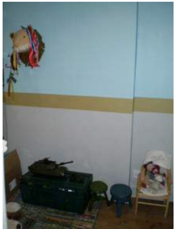
Third floor front north room. Original chimneybreast - Low Significance. Fireplace removed - Harmful alteration.
