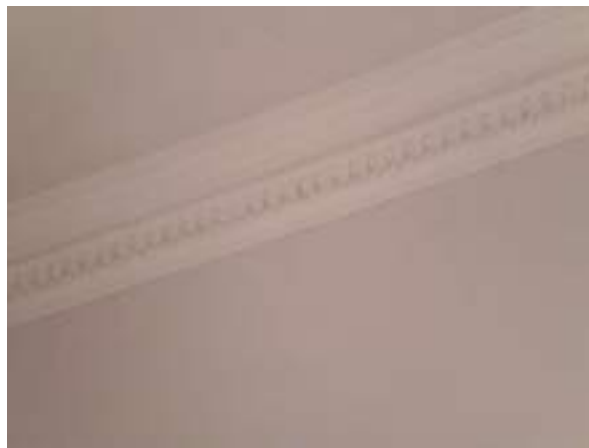
Ground floor front room. Non-original period cornice - No Significance. Medium architectural merit. Worthy of retention.
