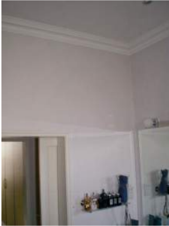
Second floor rear room. Modern partition and sliding door - harmful modern alteration. Modern period ceiling cornice - No Significance. Medium architectural merit.
