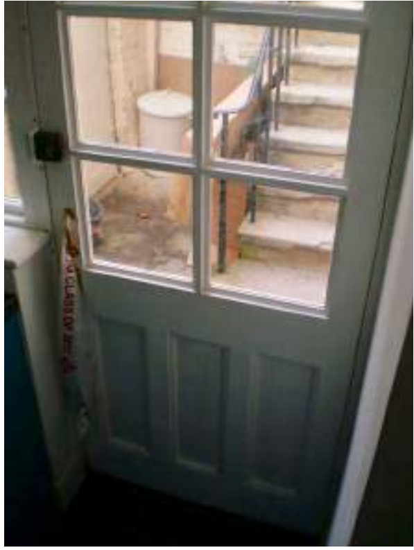
Basement front entrance door. No Significance. Harmful modern alteration.
