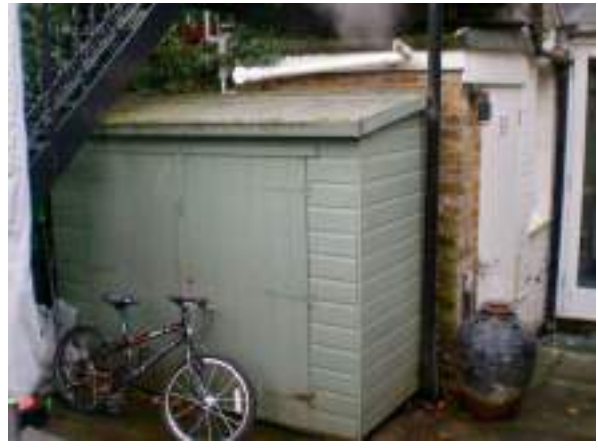
Modern single-storey brick extension and boiler flue and modern shed. No Significance. Harmful modern alterations.
