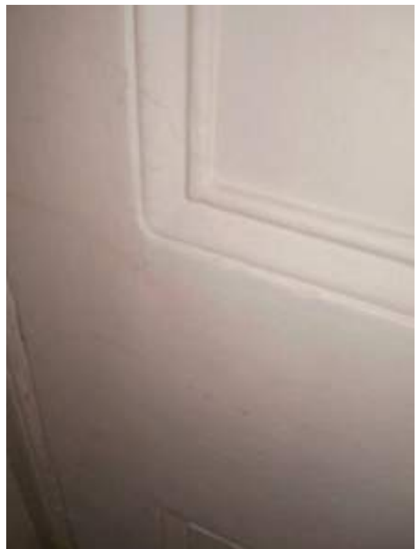
Detail of under-stair door panels; flat recessed panels with ogee bed mouldings - High Significance.
