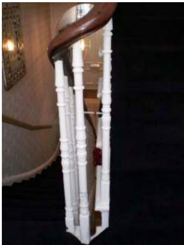
Detail of swept continuous handrail on first mezzanine level. Original feature - High Significance.
