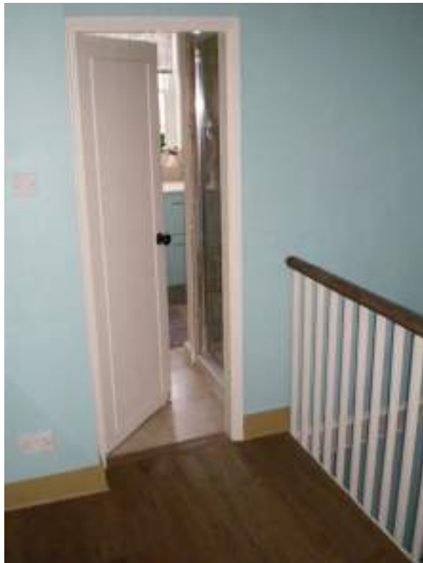
Third floor landing. Non-original door and partition wall to left - Harmful modern alterations. Original balustrade - High significance.
