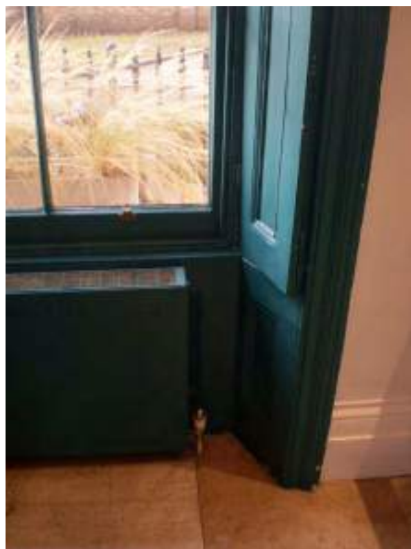
Ground floor front room. Detail of original window, shutters and architrave - High Significance.
