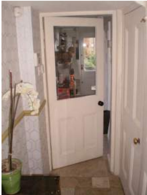
Ground floor staircase compartment. Part-glazed door to rear wing. A modern alteration - No Significance. Moderate architectural merit.
