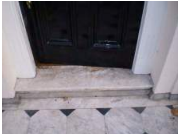
Non-original marble door step. No Significance. Harmful modern alteration.
