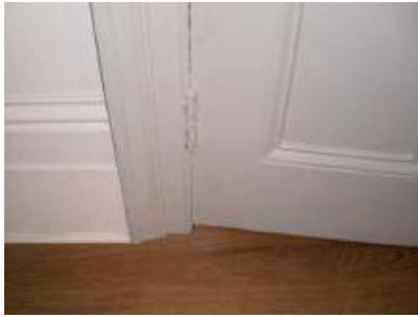
First floor rear room. Detail of door architrave and panels. - High Significance.
