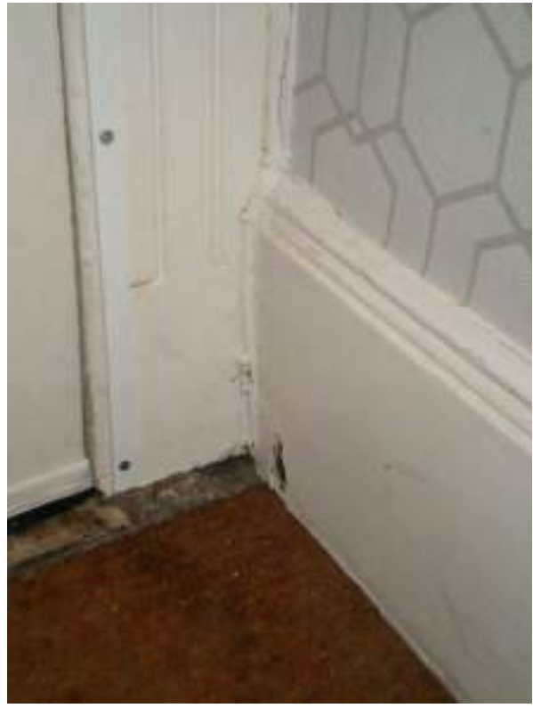
Front entrance hall, original moulded door frame and skirting board - High Significance.
