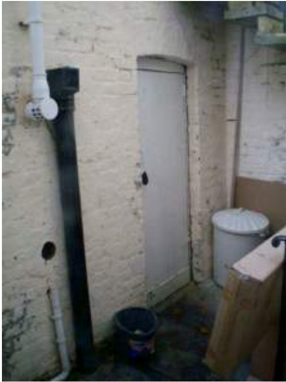
Front basement lightwell. Original door to vault - Low Significance. Modern boiler flue - harmful modern alteration.
