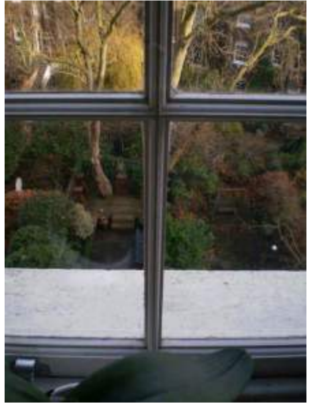
Third floor rear south bathroom window. Modern replacement. Joinery mouldings do not match originals.
