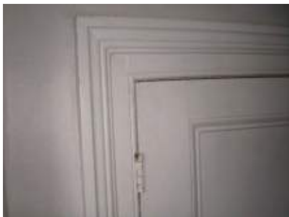
Ground floor rear wing. W.C. door architrave and panel details. Original - Medium Significance.
