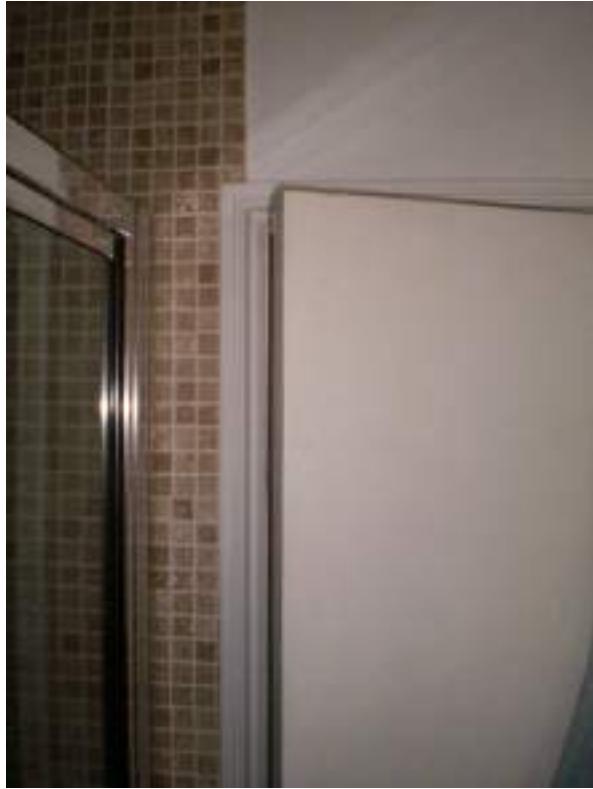
Third floor rear south bathroom. Modern architrave - No Significance. Flush door - harmful modern alteration.
