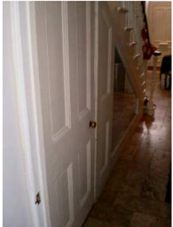
Ground Floor staircase compartment. Original door to basement stairs and surviving panelled partition - High Significance. Glazing inserted and panelling removed - harmful modern alteration.
