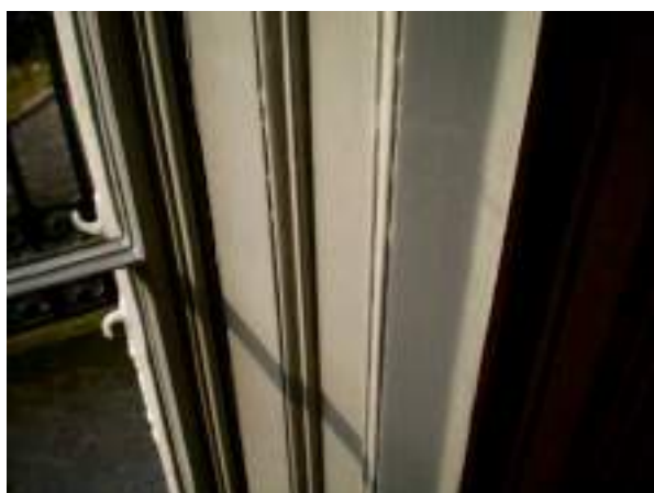
First floor front room. Original lamb's tongue window frame and shutter joinery details - High Significance.
