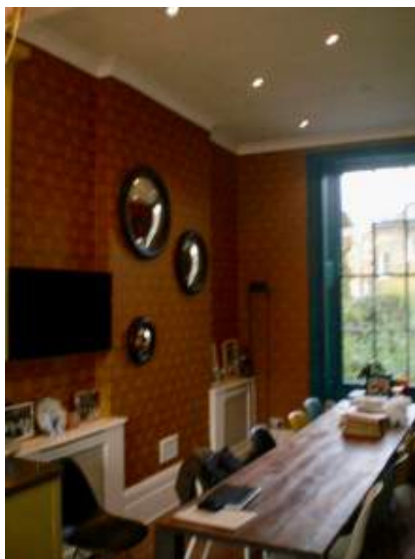
Ground floor rear room. Fireplace removed - harmful modern alteration. Modern radiator cabinets in recesses - No Significance.
