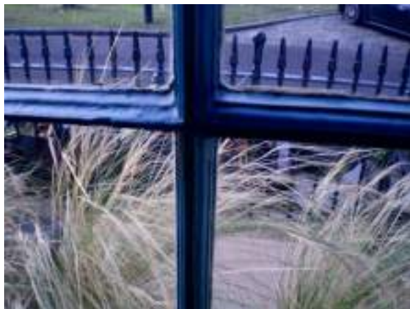
Ground floor front room. Detail of window joinery. Original lamb's tongue moulding glazing bar on left, later long ovolo replacments in centre and right.
