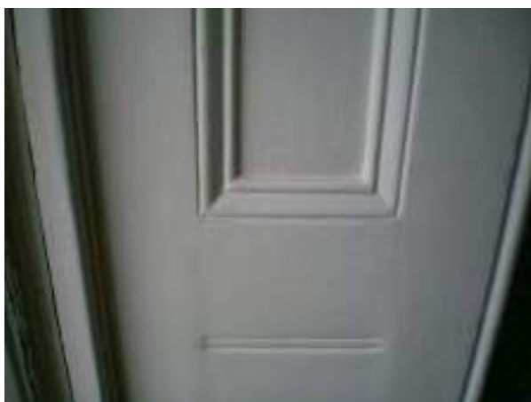
Detail of panelled lining of French doors on first mezzanine landing with flat recessed panel and ogee bed moulding above and flush panel with butt and bead moulding below - High Significance
