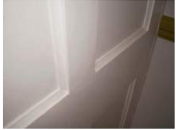
Detail of airing cupboard door - inappropriate panel moulding.
