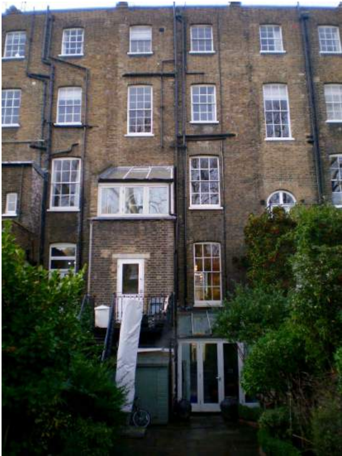
Rear Elevation. Overall, Medium Significance. Untidy pipework - harmful alteration.
