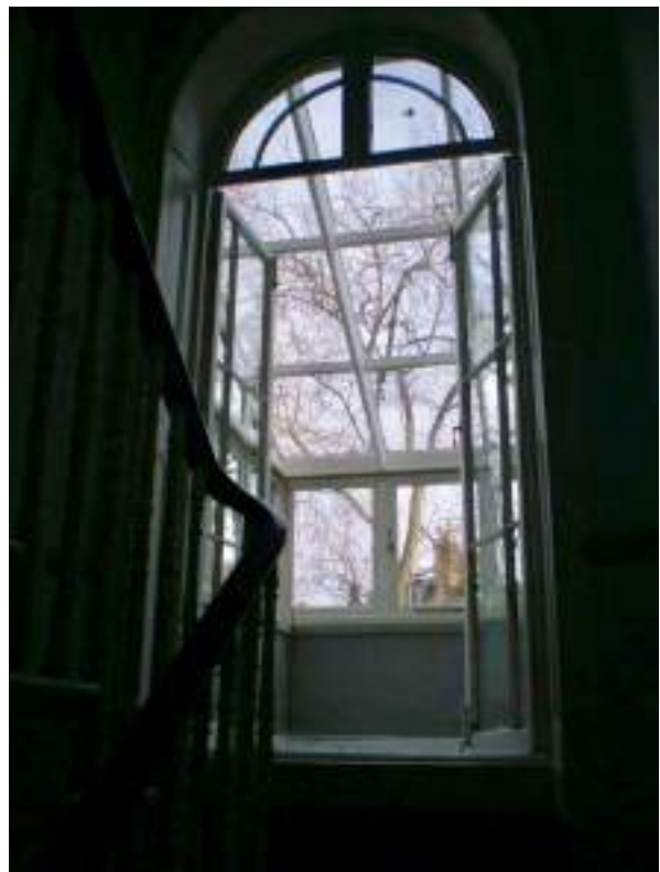
First floor half-landing. French doors leading to terrace and conservatory. Original feature - High Significance.
