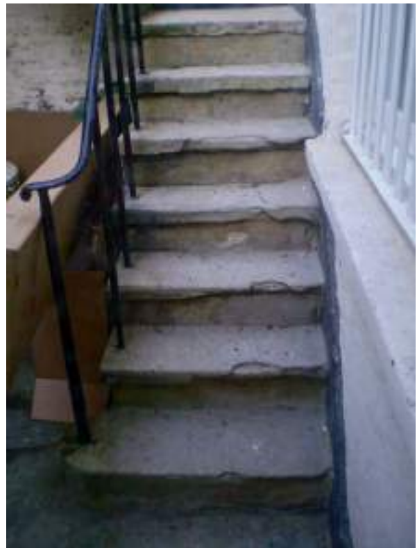
Front Basement lightwell. Original York stone steps and railings, steps patched with cement. High Significance.
