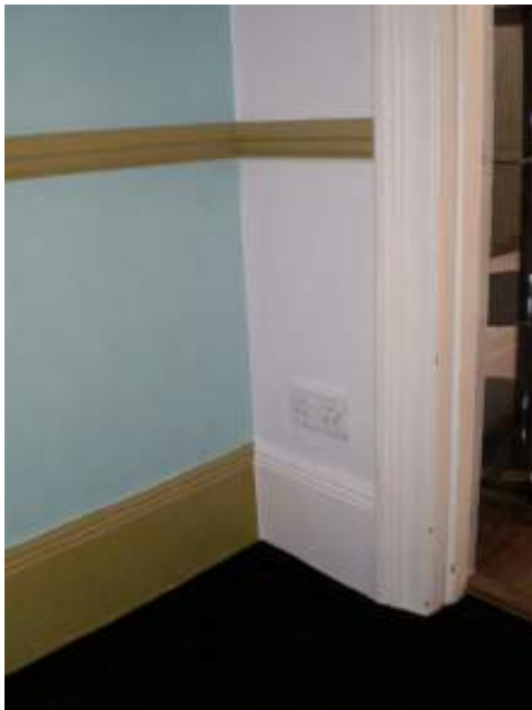
Detail of first floor landing original skirting board, door architrave - High Significance. Dado rail, later alteration - No Significance.
