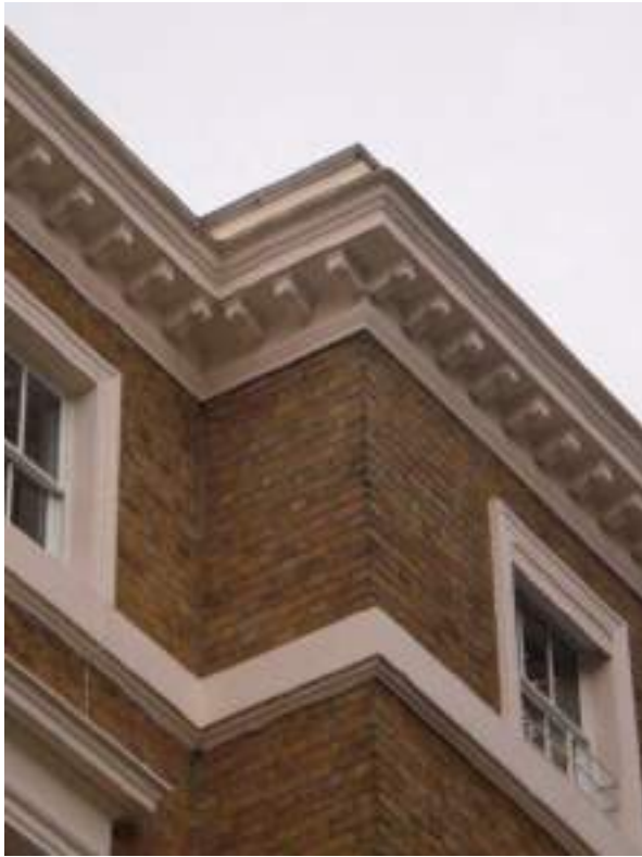
Parapet cornice with modillions, plain storey band below third floor windows. High Significance.
