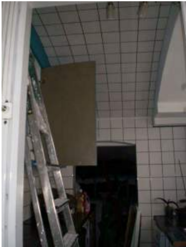
Basement entrance lobby under front door bridge landing. Negligible Significance
