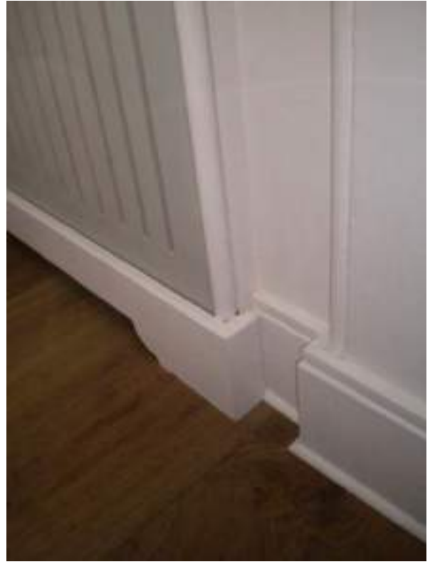
Second floor front room. Non-original skirting boards, a near match - No Significance.
