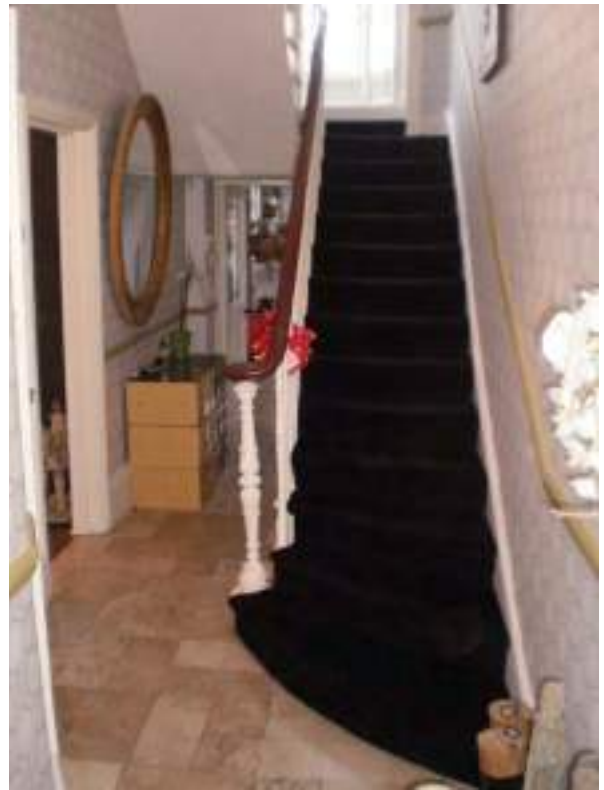
The staircase and corridor. Original plan form. High Significance. Stone floor tiling - harmful modern alteration.
