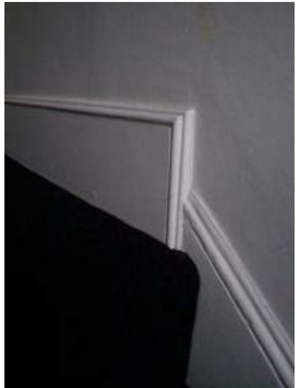
Detail of second floor stair's original skirting board - High Significance, and second floor landing's modern skirting board not an accurate match - No Significance.
