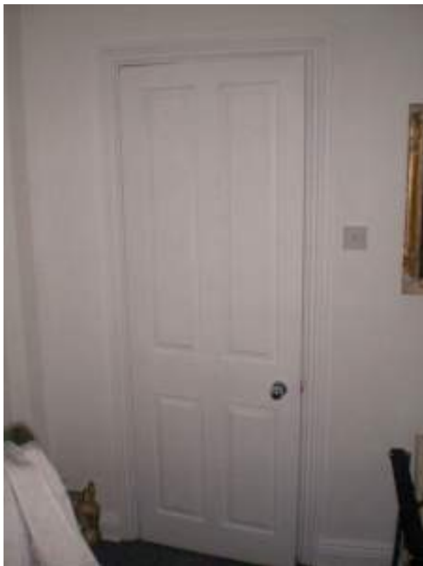
Basement front room. Modern four-panelled raised and fielded panelled door. No Significance. Harmfull modern alteration.
