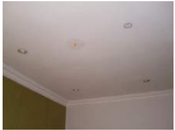
Second floor front room. Modern period ceiling cornice - No Significance. Medium architectural merit. Recessed spotlights - Harmful modern alteration.
