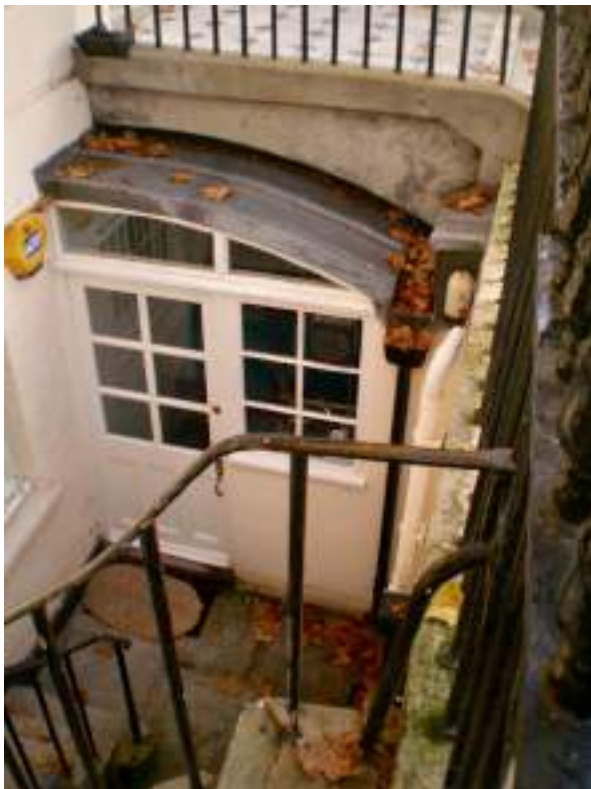
Front Basement Lightwell Non-original door & window infill under bridge - No Significance. Harmful modern alteration
