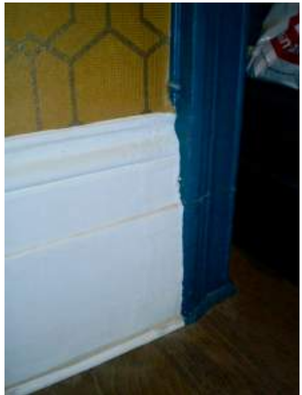
First floor rear room. Detail of original window architrave and skirting board - High Significance.
