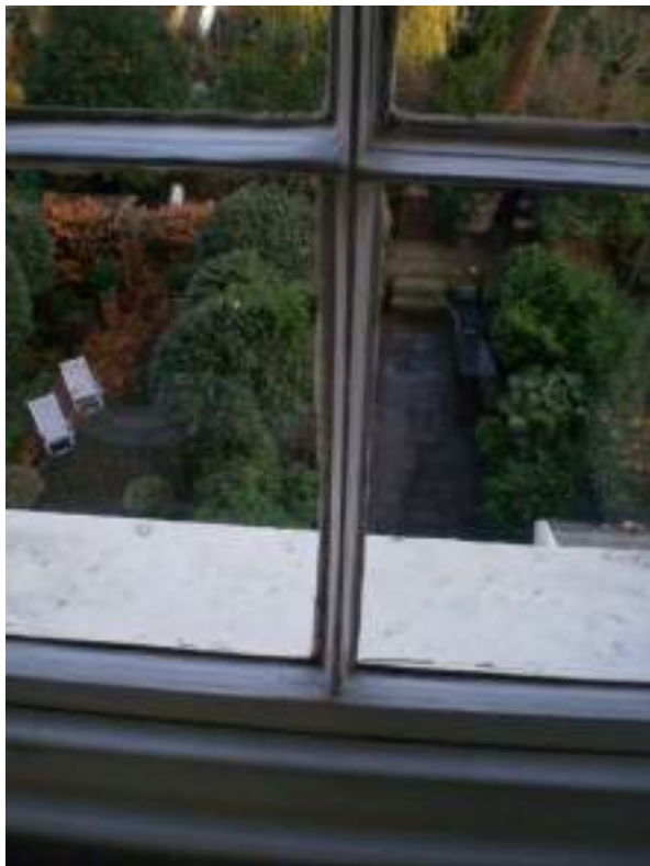
Second floor rear room. Original sash frame with lamb's tongue mouldings - High Significance.
