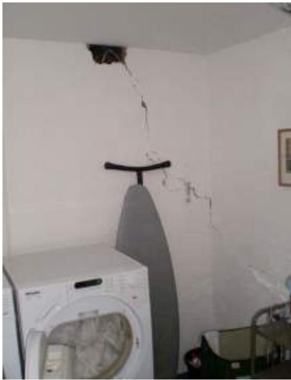
Rear wing, basement. Crack in rear and south wall.
