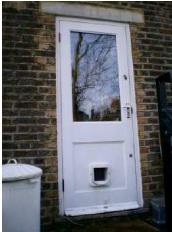
Modern door and concrete lintel. No Significance. Harmful modern alterations.
