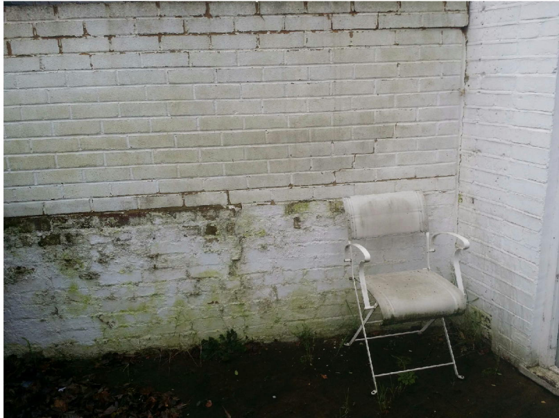
Photo two: shows left hand boundary wall with cracking. Lower section is 225 mm thick brickwork; the upper more modern section is 100 mm thick.
