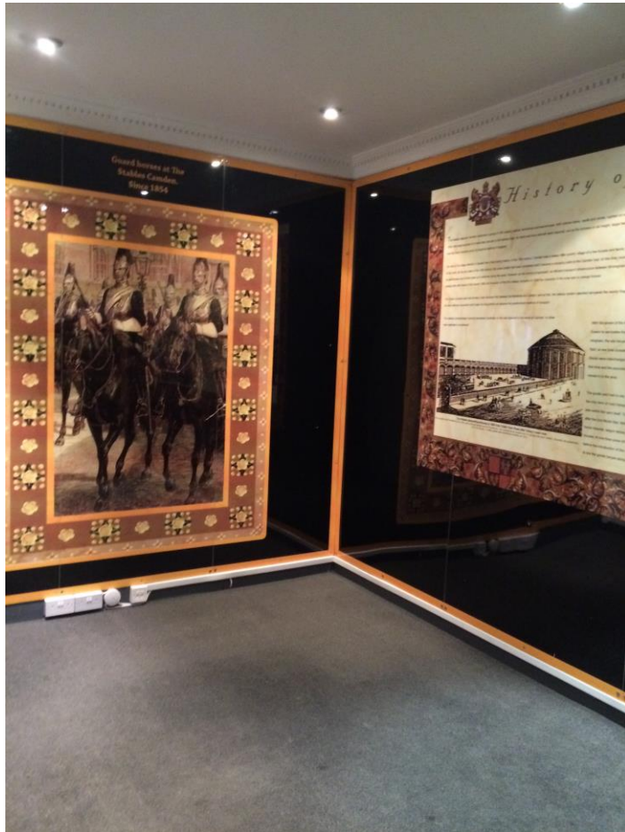
Figure 7: Tack Room: first floor: north bay. Modern wall linings, partitions and suspended plasterboard ceiling to be removed.
