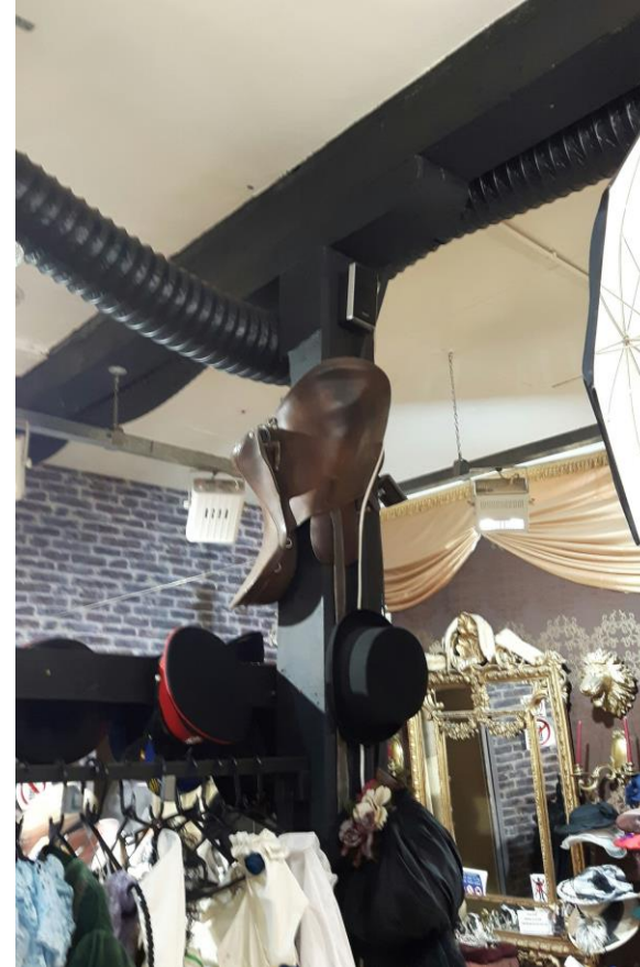
Figure 6: Tack Room: ground floor: north bay. The partitions and wall linings are modern and to be removed. The timber first floor structure and column are original.
