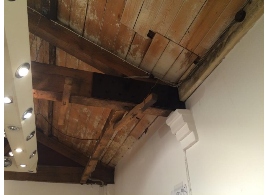
Figure 10: Tack Room: first floor: middle bay. The timber sarking boards are to be repaired and replaced where necessary to match the original existing boards and painted white to recall the likely original lime/white wash finish. The timber trusses and purlins are to be left unpainted showing the natural grain of the wood.
