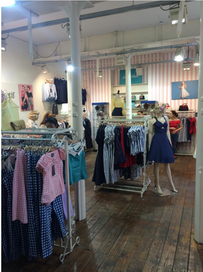
Figure 5: Tack Room: ground floor: middle bay. The partitions and wall linings are modern and to be removed. The timber floorboards are to be replaced and the entire ground floor made level throughout.
