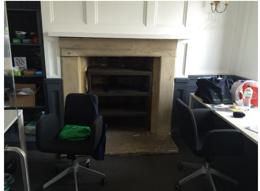
Figure 8: Tack Room: first floor: north bay. The fireplace and surround is to be retained; the panelling is modern and to be removed.
