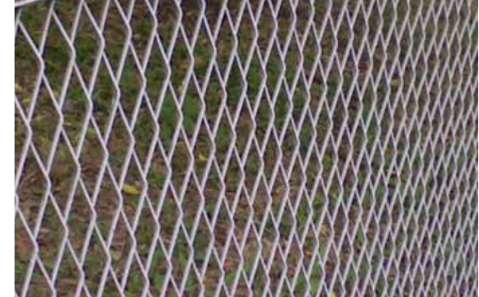
Galvanized steel 'Carl Stahl' mesh balustrade
