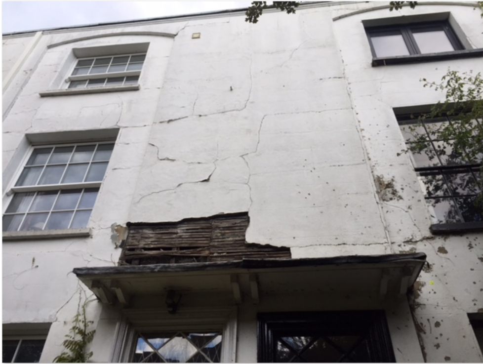
Photo 3: Crumbling render to front elevation, taken on 11/10/2016.
