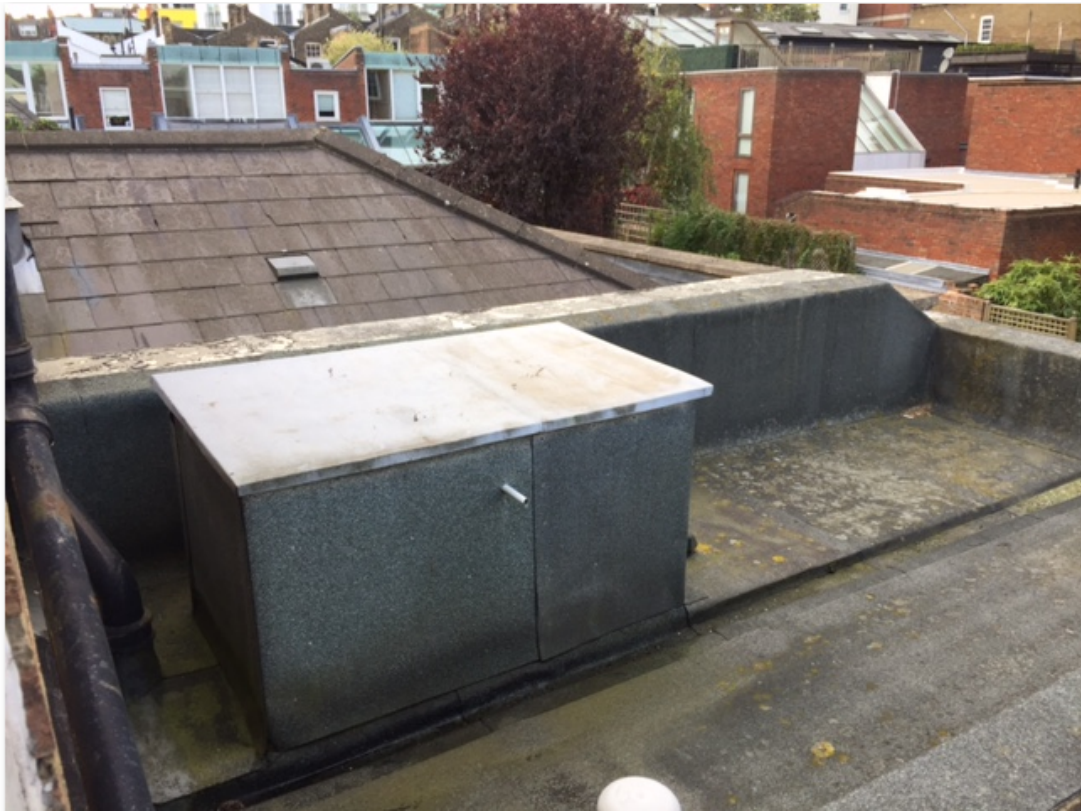
Photo 7: View across roof of existing extension of 3 storey extension to rear of no.43
