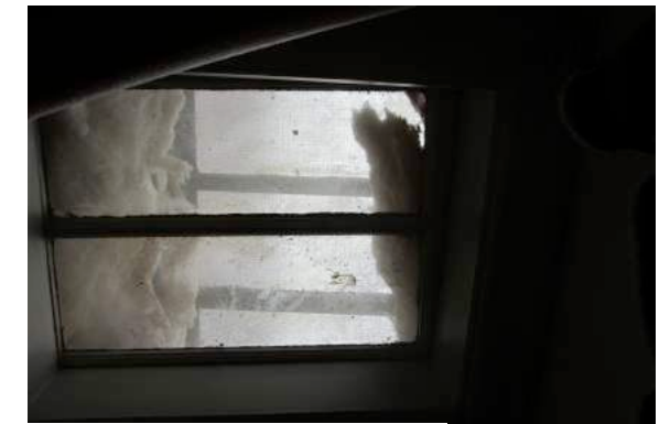
Dilapidated rooflight from inside
