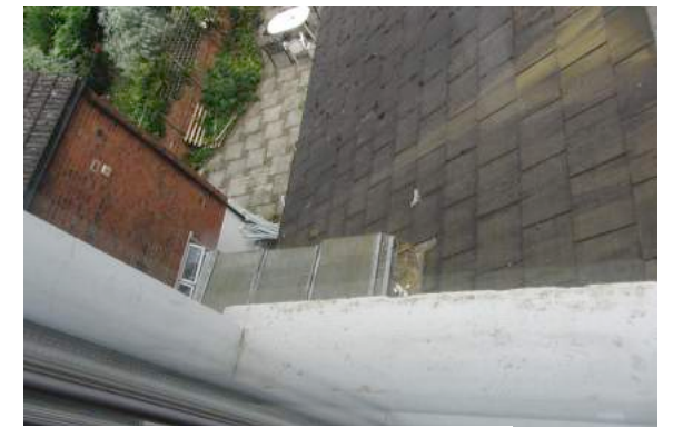
Dilapidated rooflight - to be removed
