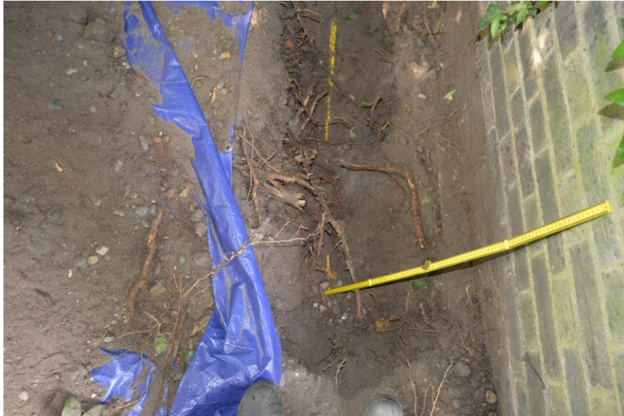
Photograph 6 The roots diverting at the root barrier interface.
