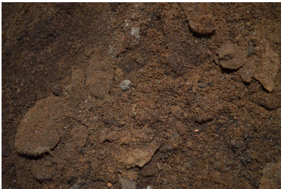
Photograph 5 Sand found at below foundation level 800mm.
