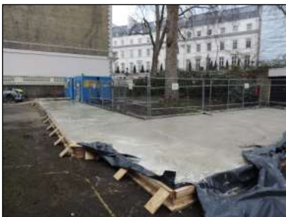
Ground protection image 1: poured concrete slab ground protection outside of CEZ fencing which is strong enough to support construction traffic and a piling rig.
