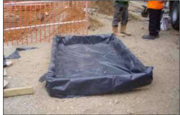
Pollution image 2: Soil bunding or a supporting framework covered in heavy-duty plastic sheeting is essential where there is a risk of spillages contaminating RPAs. This specifically applies to cement mixing areas and vehicle washing facilities.
