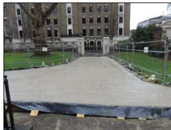
Ground protection image 2: Concrete ground protection over an existing drive to prevent damage to roots below the drive by heavy construction traffic.
