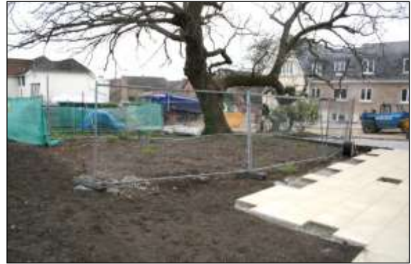
Landscaping image 2: This tree had tarmac parking within its RPA that was removed and replaced with an organic mulch near the trunk and limited no-dig surfacing on the outer edges of its RPA.
