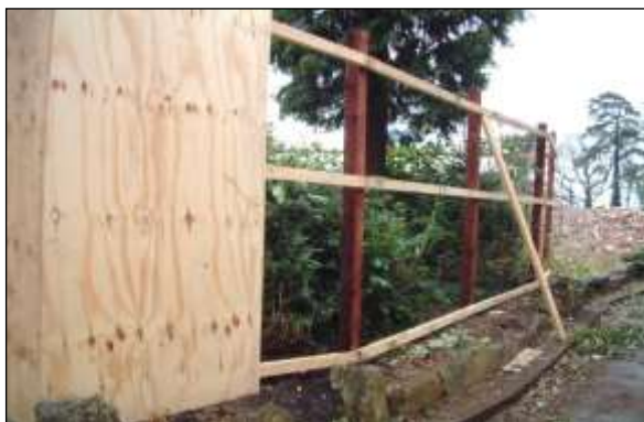
Fencing image 4: Board specification on secure wooden posts is a suitable alternative to the standard braced scaffold design.
