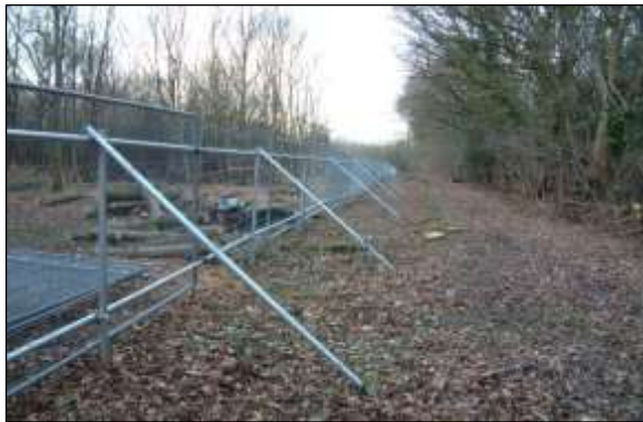
Fencing image 2: Heras fencing wired to scaffold braced posts is a robust and effective interpretation of the BS specification.
