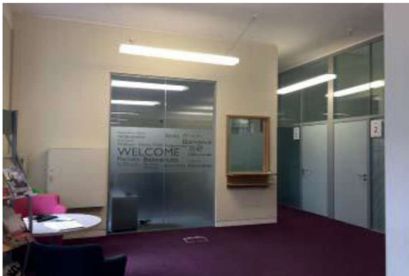
Photo 3. Partition wall dividing the reception of RAC and the office space and meeting room - To be removed
