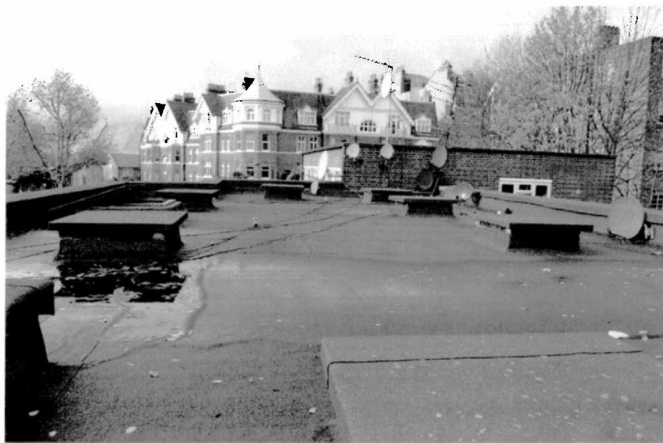
Showing the Edwardian block of flats beyond. Roof of Block 7-12 standing east looking west.
