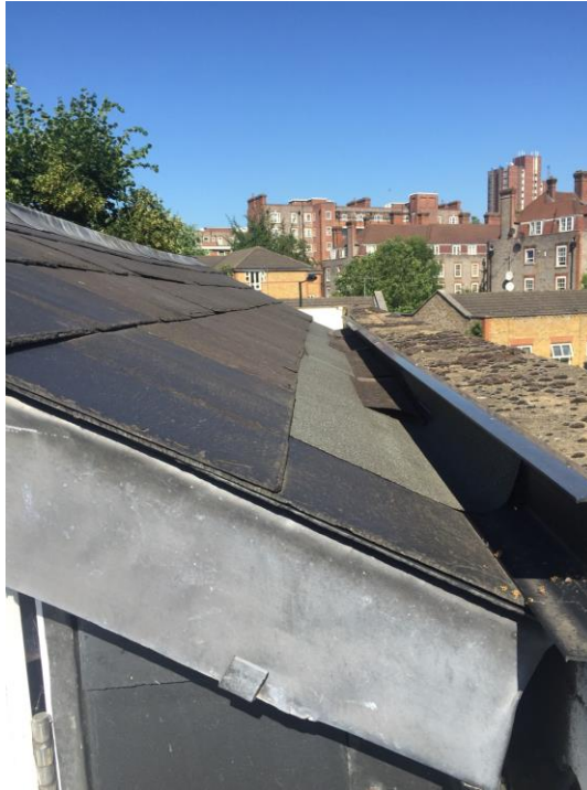
Existing poor quality mansard roof extension.
