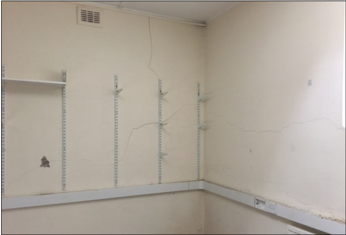
Figure 1: Damage to masonry in close proximity to tree located in court yard
