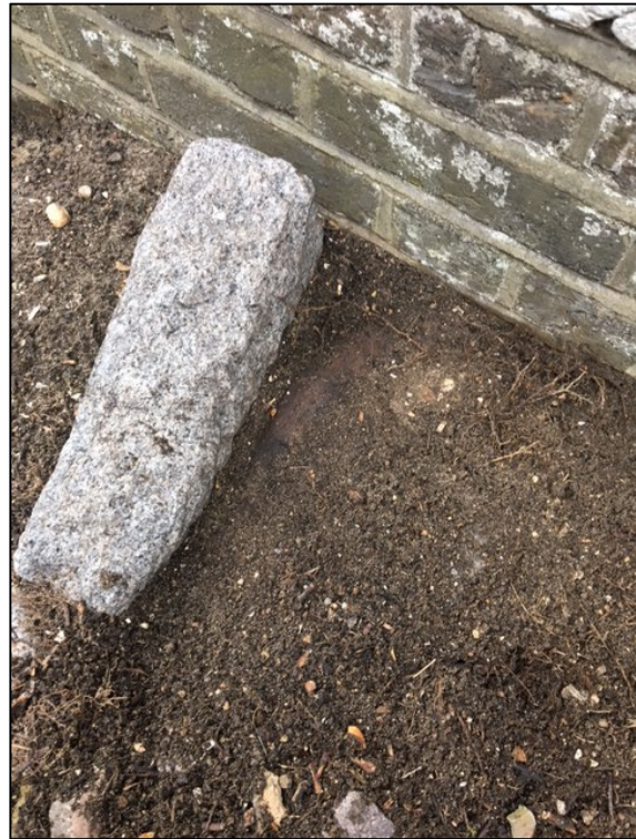
Figure 3: Root growing directly toward damaged area of wall
