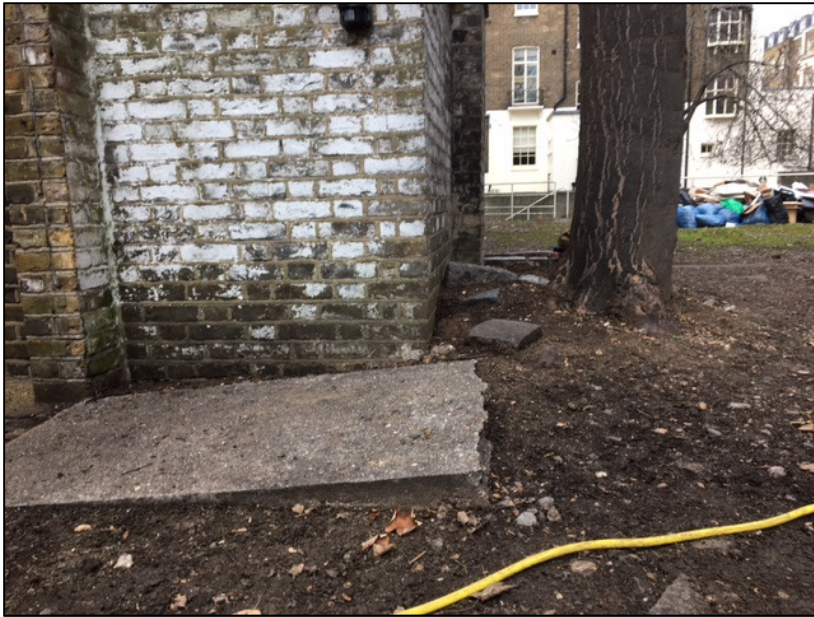
Figure A: Tree in close proximity to property pushing bricks towards wall
