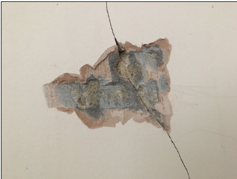
Figure B: Internal damage to wall within property
