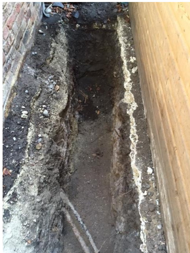
Photograph #4 – showing the second stage of the excavation to a depth of 700mm with no roots encountered
