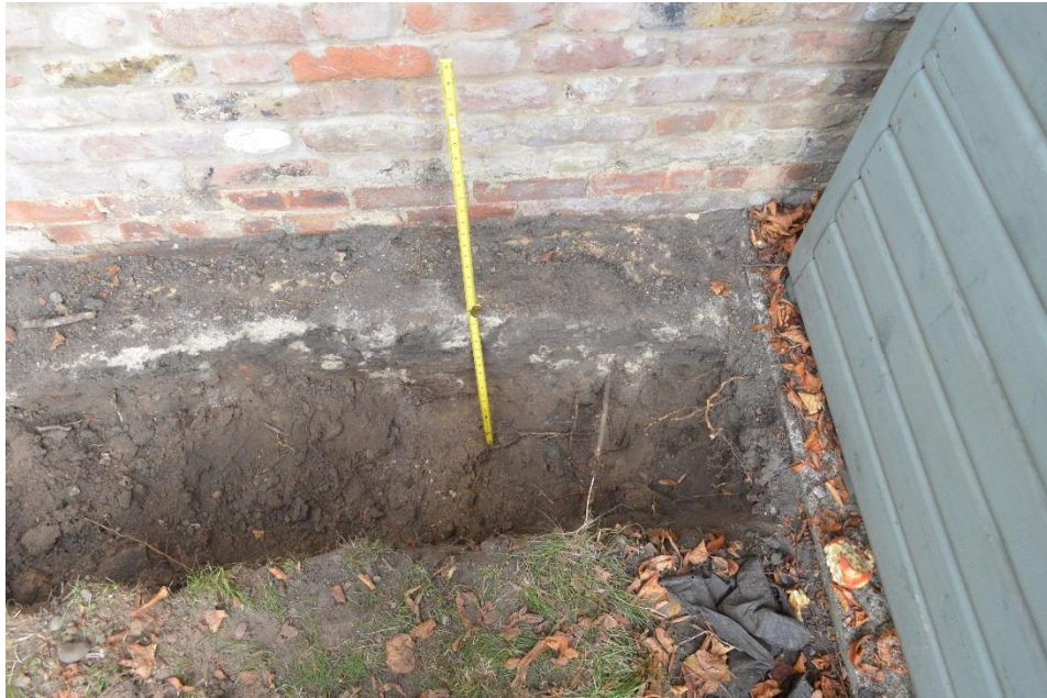
Photograph #3 – Showing the first stage of the excavation to a depth of 650mm with only one cypress root found
