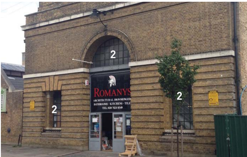
Front Entrance (Revised on 15/08/07) - Highlighted windows to be renovated - retaining the original metal frames and replacing individual panes where damaged.
