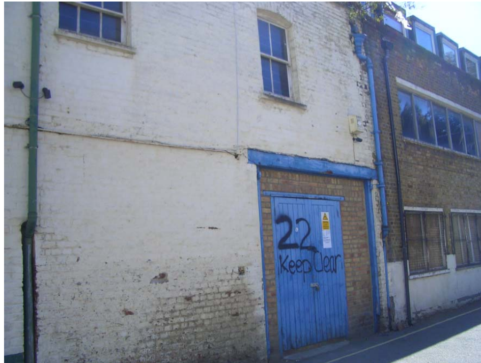
Figure 4: Partial view of front elevation of property showing hard-standing and rain water pipes.
