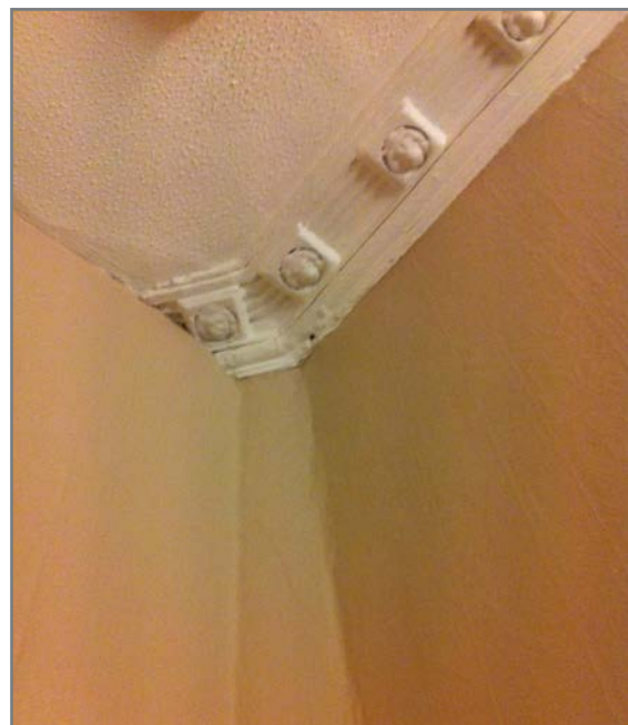
Remains of Original Cornice
