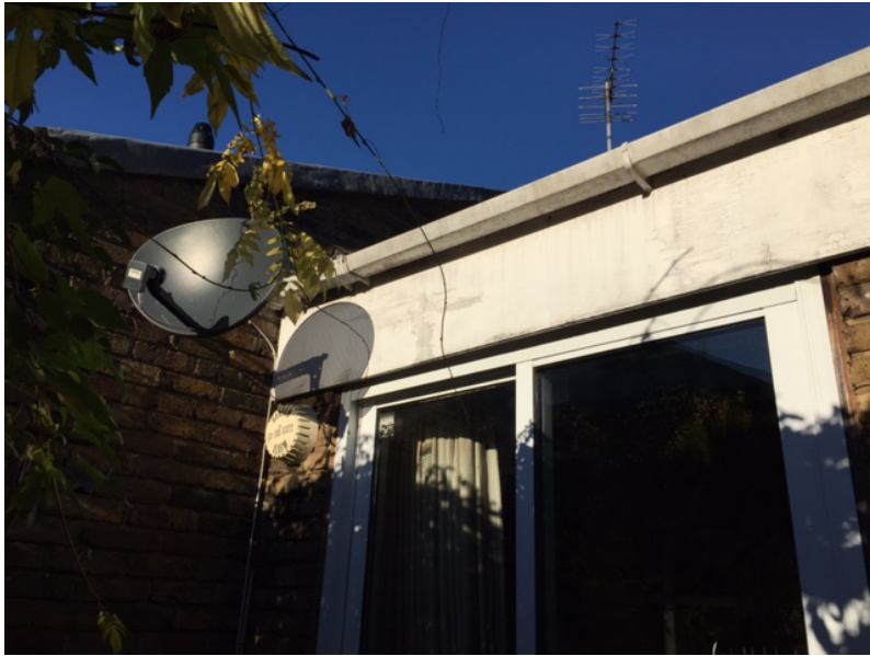
Photo 7 (above): View of roof and side wall of 11 Old Brewery Mews as viewed from existing terrace
