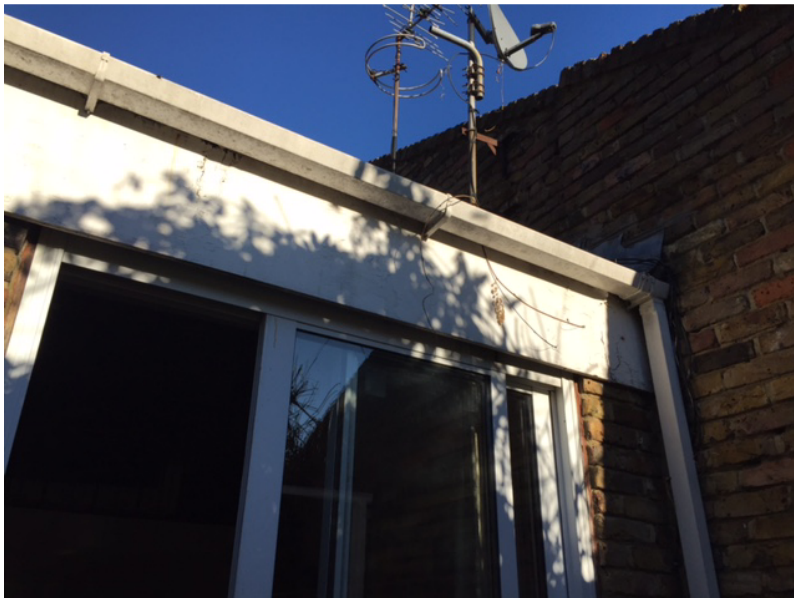
Photo 8 (above): View of roof and side wall of 9 Old Brewery Mews as viewed from existing terrace
