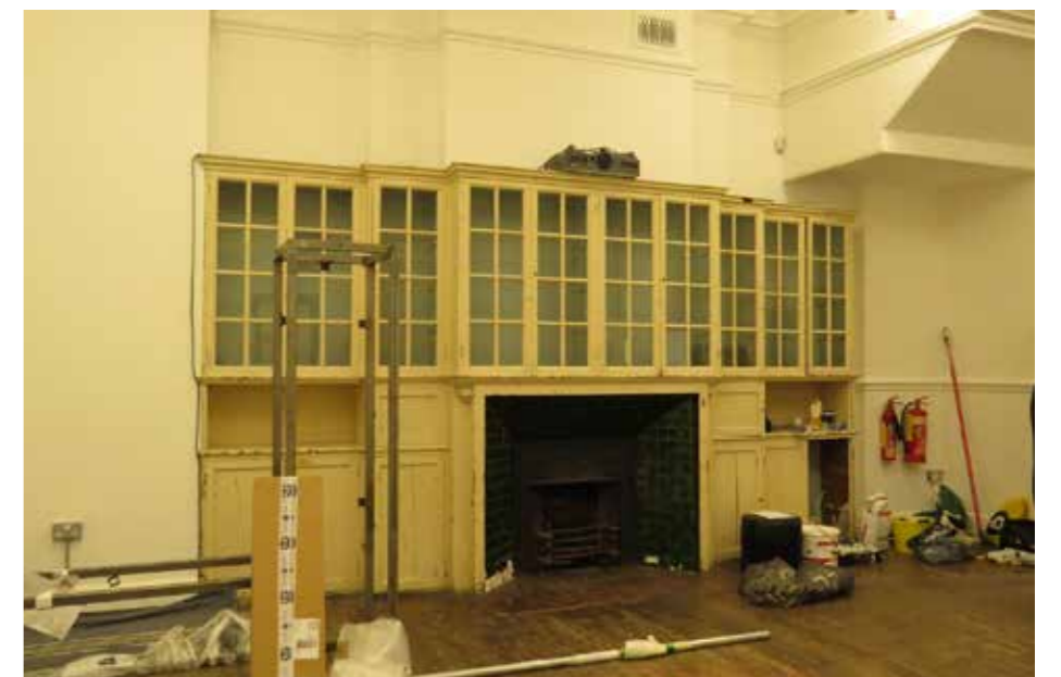
Figure 4.14 View of the fireplace in the rear room in the middle gallery
