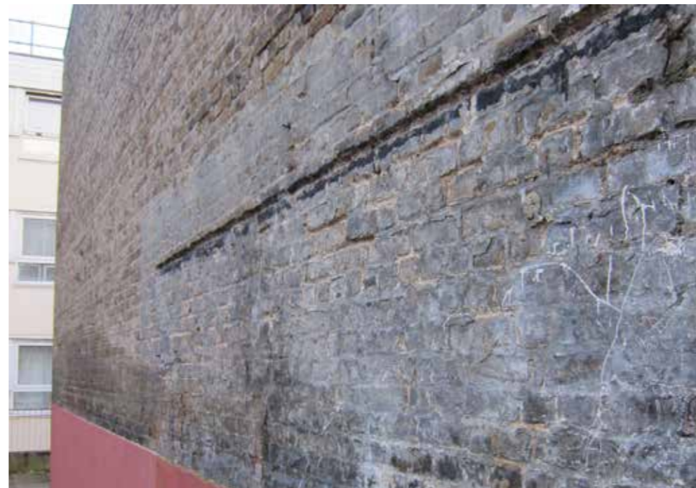
Close up showing state of brick
